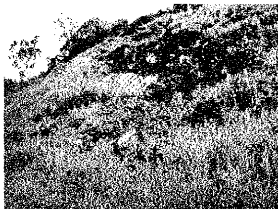
Figure 2.4.7 Wedge Slip (E-W Highway, 15.1 km)
