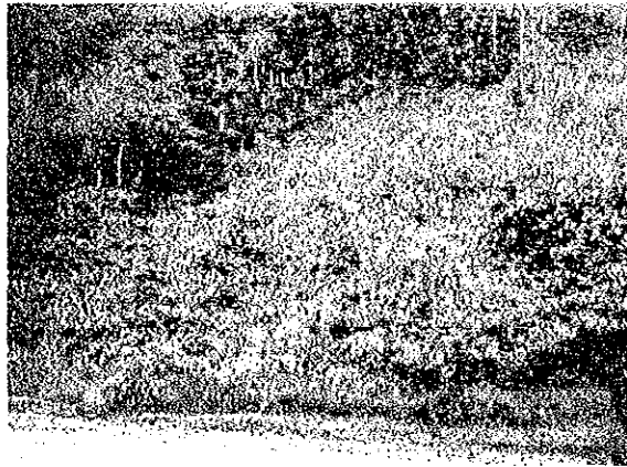
Figure 2.4.8 Rock Fall (Sabah Rd. 78.6 km)
