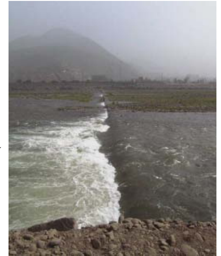
The Rimac River upstream of La Atarjea: channel widening works with concrete wall for groundwater recharge.
