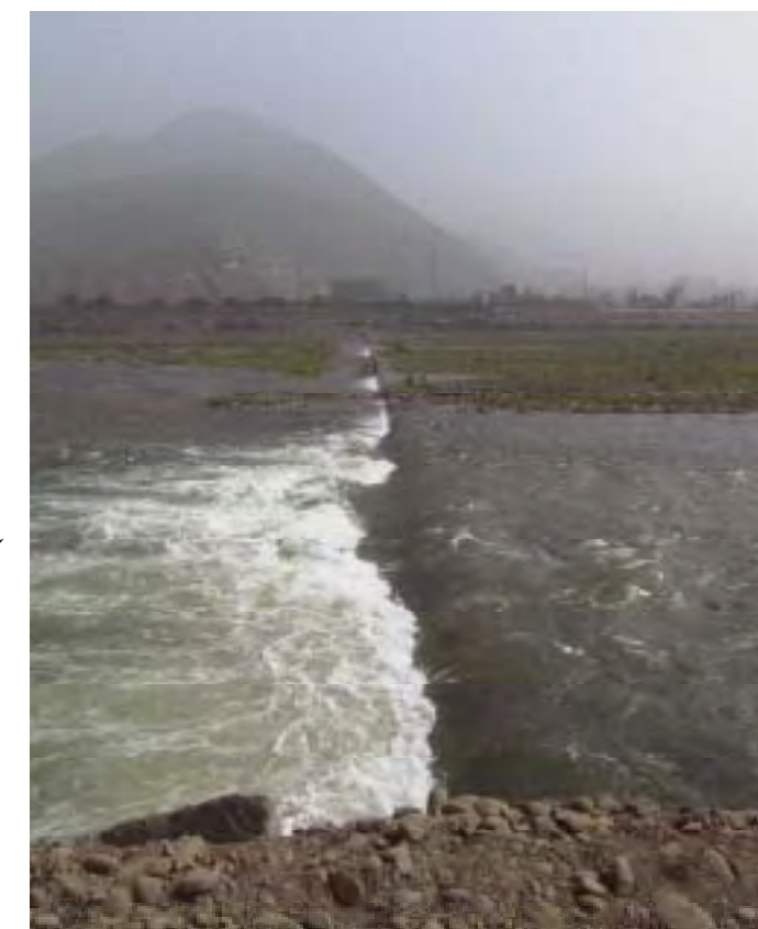
The Rimac River upstream of La Atarjea: channel widening works with concrete wall for groundwater recharge.
