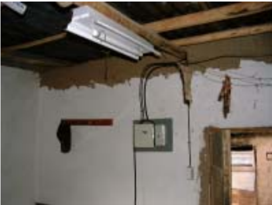
The lamp installed
