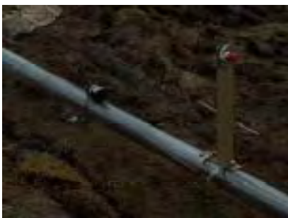
Pyranometer and Air Pressure Sensor
