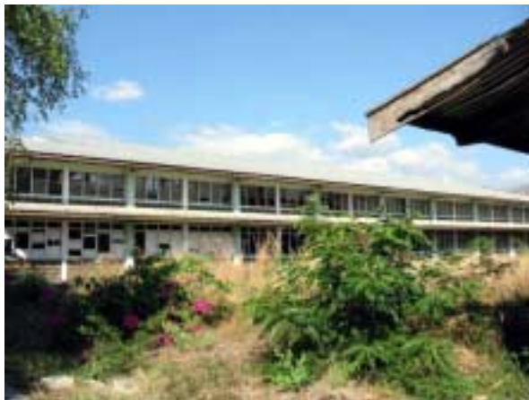
Exterior View : Aluminum sash and glasses are broken.
