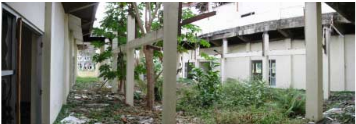
Ground floor Corridor : Roof and Ceiling was broken by fire
