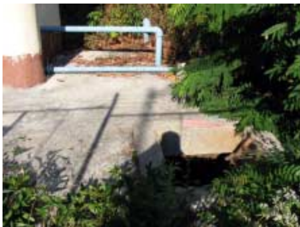
Reservoir: broken and mud settling
