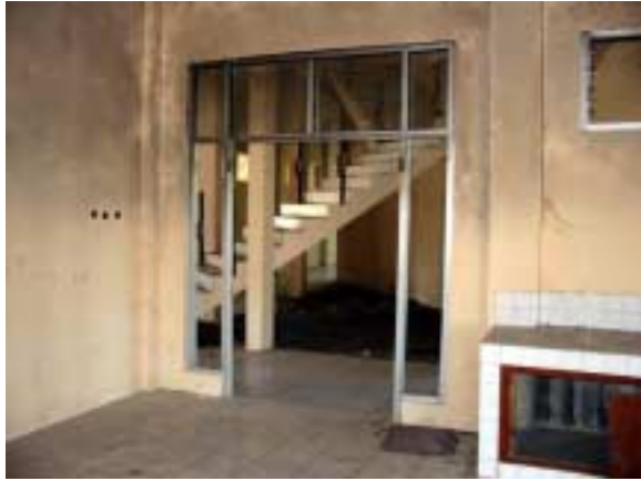
Laboratory : Door panels are missing and aluminum door frame is broken.
