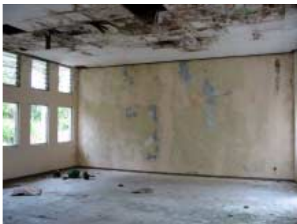
Lecture Room : Water leakage on the ceiling and cracks on the wall.
