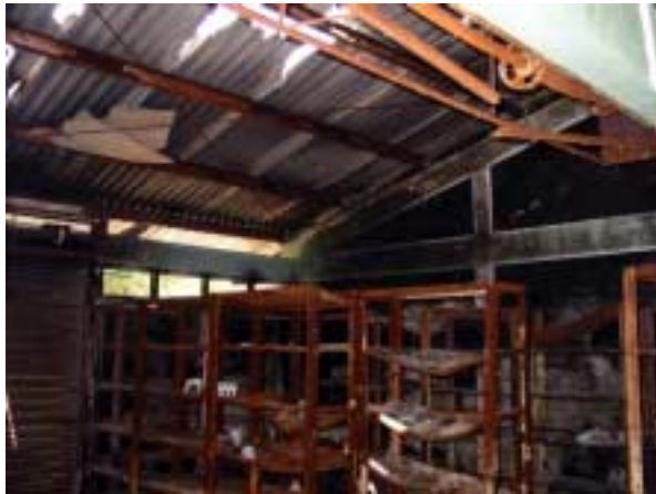
Lower part of Workshop : Fire damage of the ceiling and roof .
