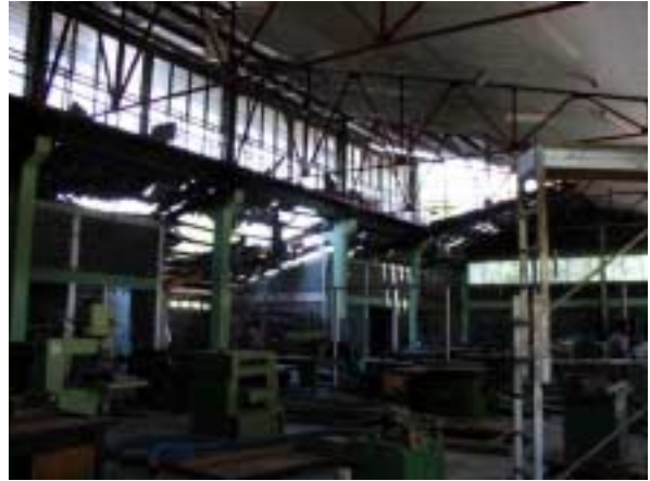
Workshop Interior View : Damaged wall and roof .
