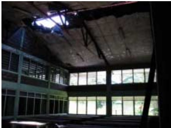
Workshop Interior View : Ceiling and roof were broken by fire.
