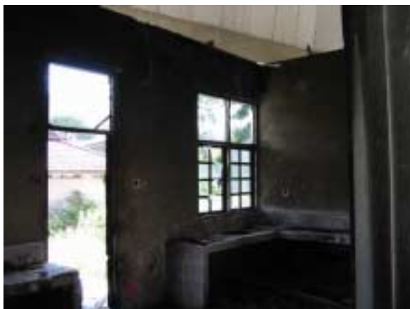
Kitchen : Fire damage
