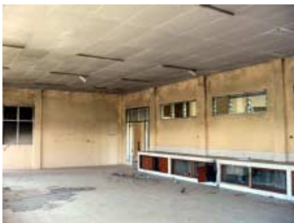
Laboratory : There are some fire damage.
