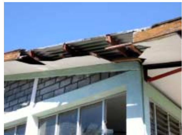
Exterior View : Damaged roof.
