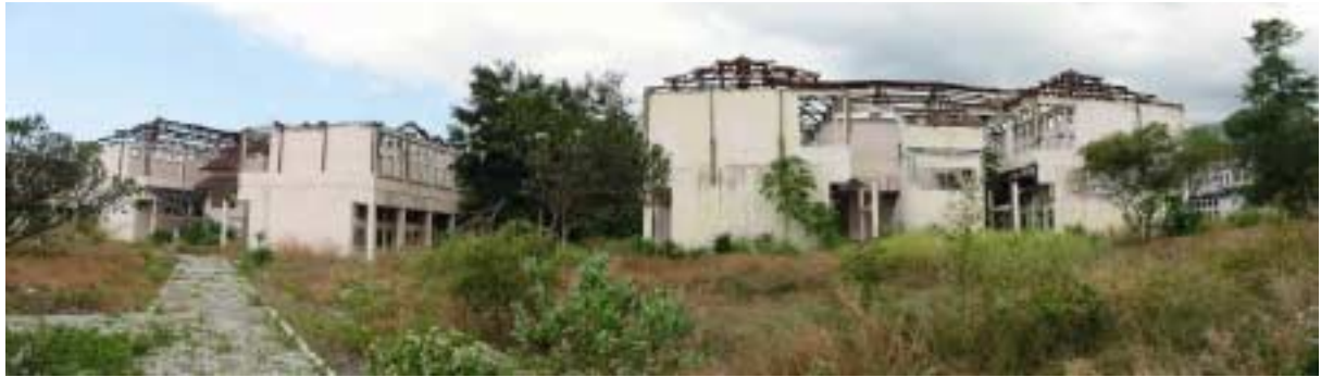
Lecture Building B · C , Panorama view : Both roof is burnt.
