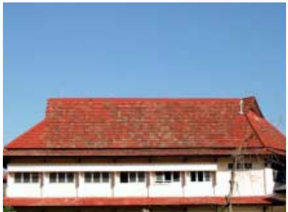
Roof: Several roof tiles are missing.
