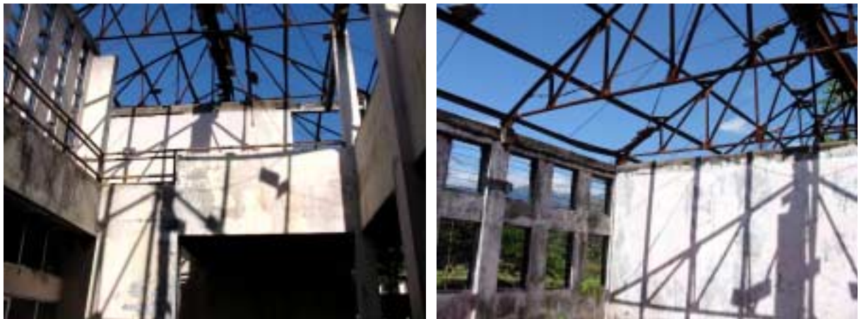
View from the Entrance Hall to the roof: Roof is completely burnt by fire.
