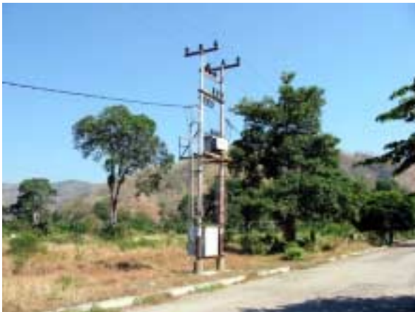
Transformer on electric pole
