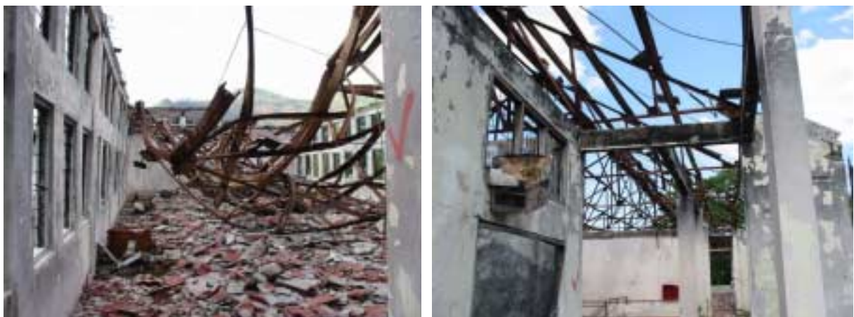
Second floor : The Roof is completely burnt by fire.
