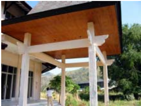
Poach : No damage by fire.
