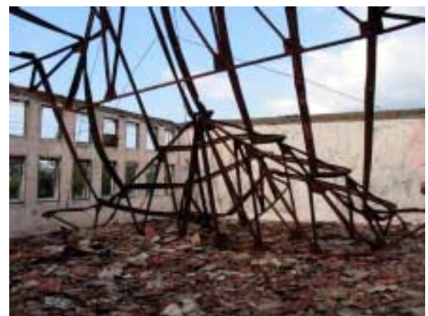
1 st floor classroom Fallen steel truss
