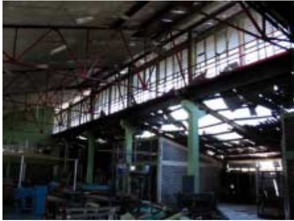
Workshop Interior View : Lower part of roof was burnt .
