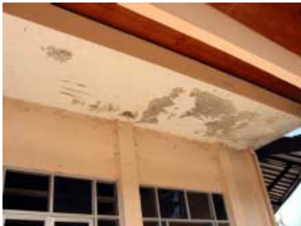
Entrance Eaves : Reinforced bars are exposed.
