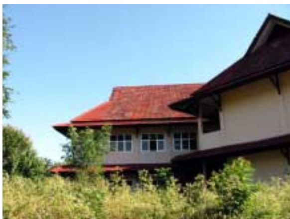
Roof: Several roof tiles are missing.
