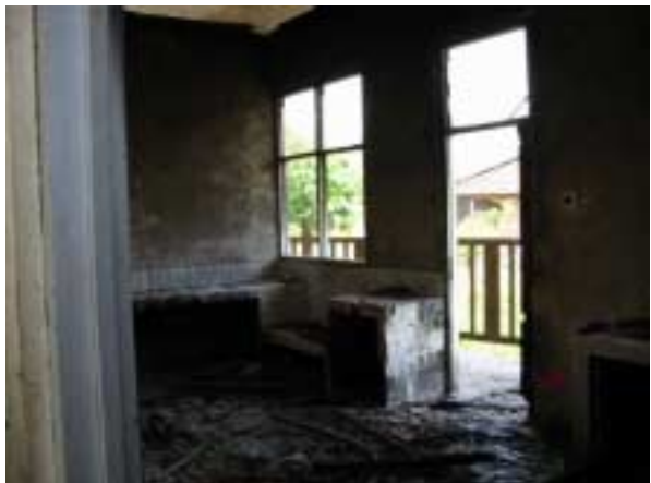
Kitchen : Fire damage
