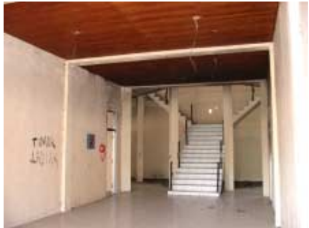
Entrance Hall : Handrail of the staircase is removed. No lighting fixtures of the ceiling.
