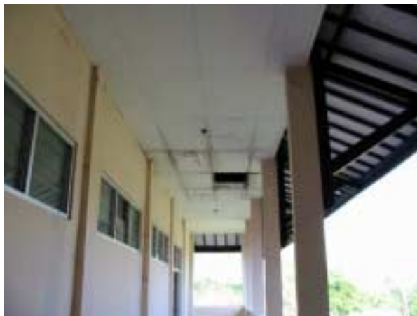
Corridor 2 nd floor : Leakage on the ceiling and cracks on the wall.
