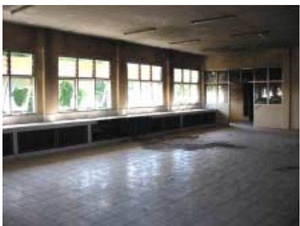
Laboratory : There are some fire damage.
