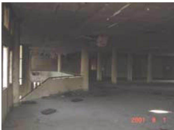
2 nd floor: Interior view, minor damage because here was few combustible material.
