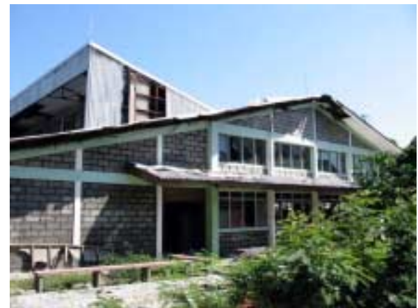
Exterior View : Damage of the roof.
