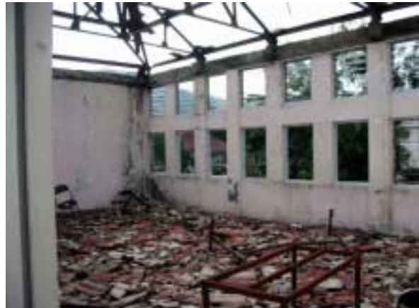
Drawing Room on 2 nd floor: Roof was burnt down.
