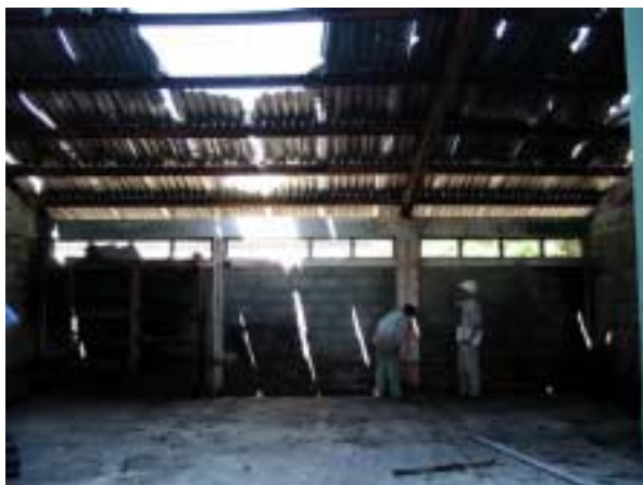
Lower part of workshop : Fire damage of Ceiling and roof .
