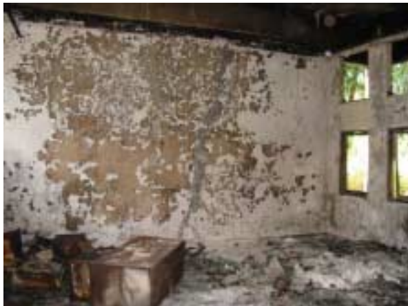
Lecture Room 1-4 : Discoloration of the mortar
