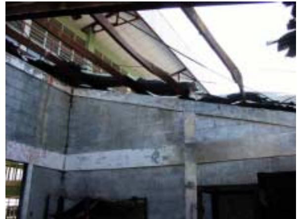
Lower part of Workshop : Roof was burnt down. Concrete surface color changed to pink.
