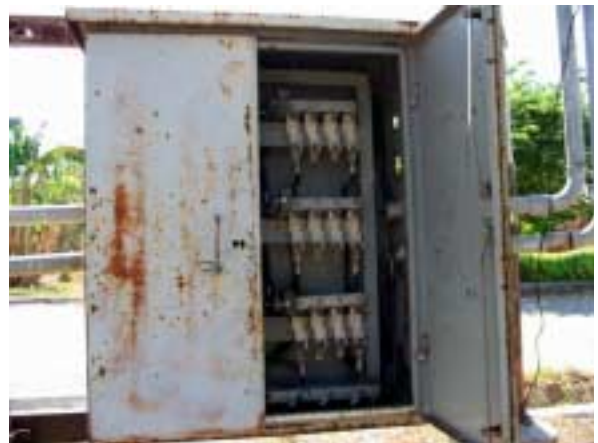
Switchboard in residential zone : broken intentionally.
