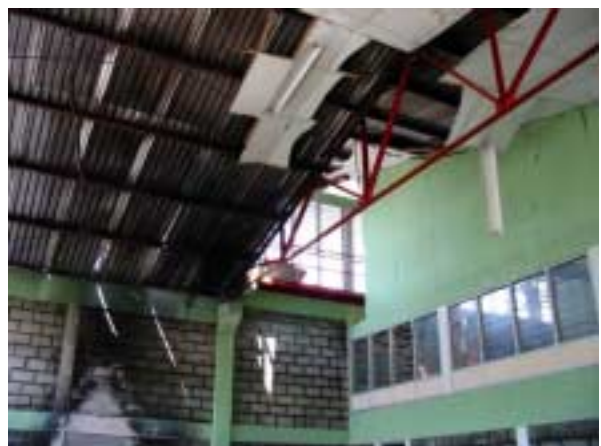
Workshop Interior View: Damaged ceiling.
