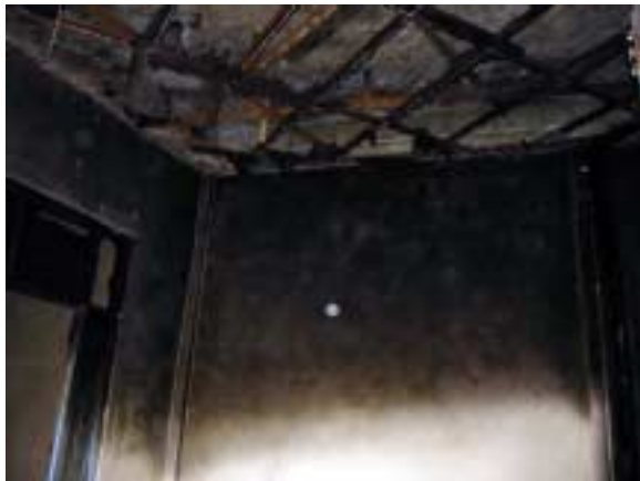
Storage : Ceiling was burnt.
