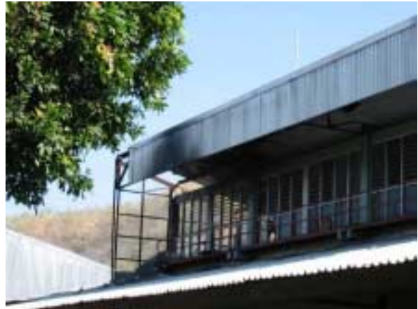
Exterior View: Roof was damaged by fire.
