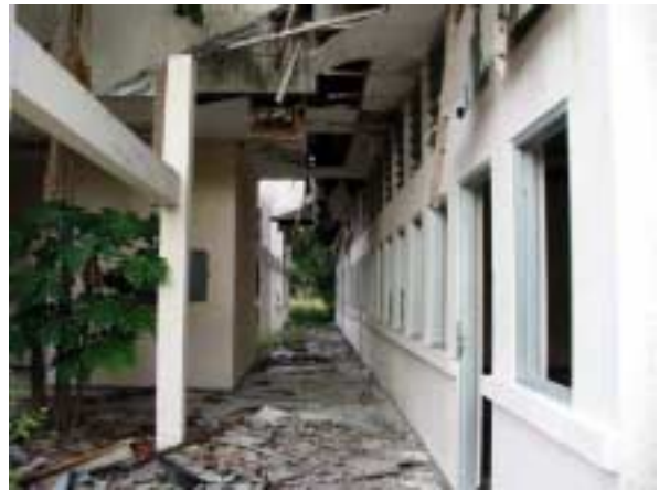
Ground floor Corridor : Ceiling was broken by fire.
