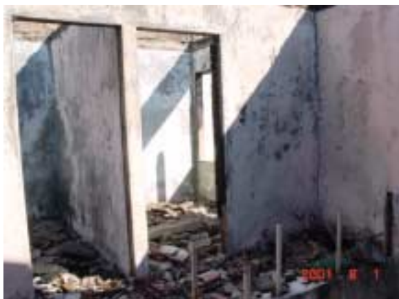
2-story house 2 nd floor Rooms were heavily burnt.
