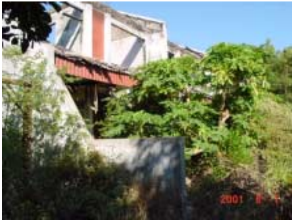
2-story house: It was totally burnt.
