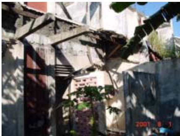
2-story house: burnt eaves
