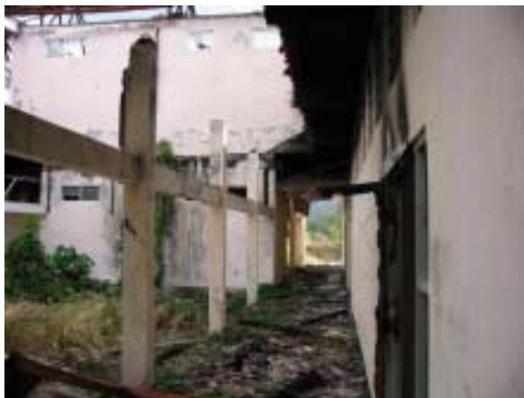
Ground floor Corridor : Roof and Ceiling is broken by fire.
