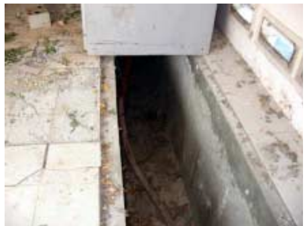
High tension panel board room : cable pit
