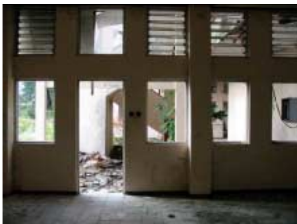
Lecture Room : Wooden door panel is missing.
