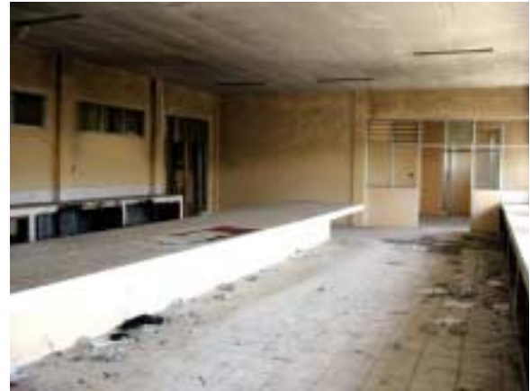
Laboratory : Floor and desk tiles are peeled off.
