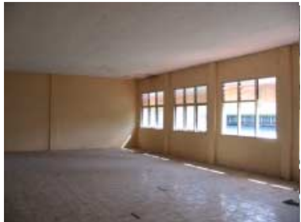
Laboratory : Water leakage on the ceiling.
