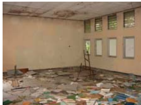
Lecture Room 1-2 : Water leakage on the ceiling, Broken Sash (All rooms of the ground floor are in the same condition, except Room 1-4)
