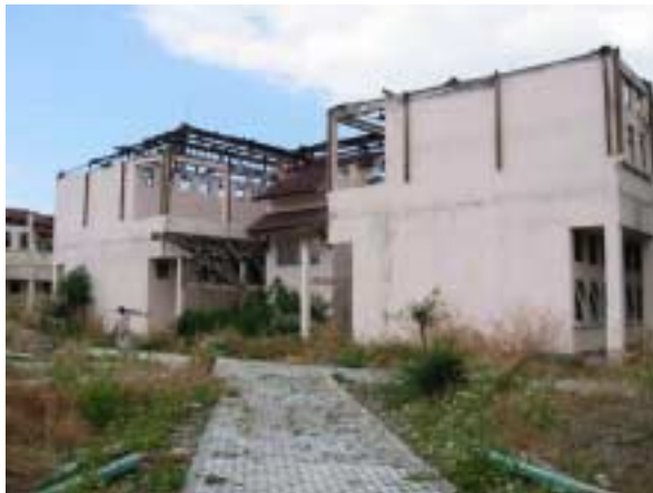
Lecture Building B : broken roof by fire
