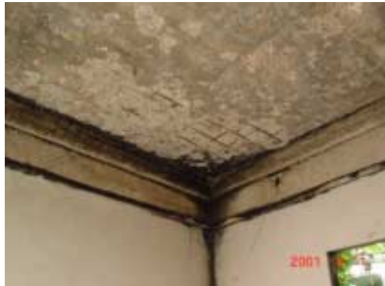
Building B Bed Room : Fire dama
