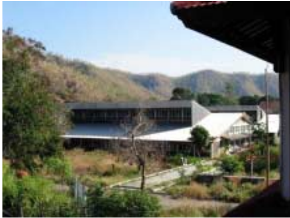
Exterior View : Fire damage on the roof.
