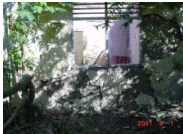
Mortar finish was peeled off.
