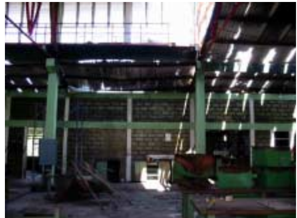
Lower part of Workshop: Damaged Roof by fire.
