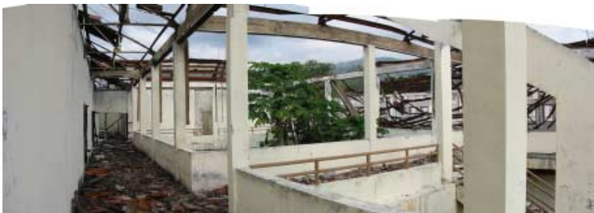
1 st floor Corridor : Roof and Ceiling is broken by fire
