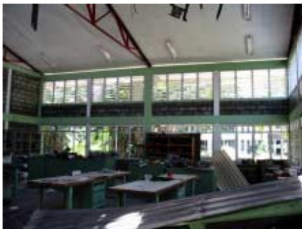
Workshop Interior View : Broken ceiling and lighting fixture.
