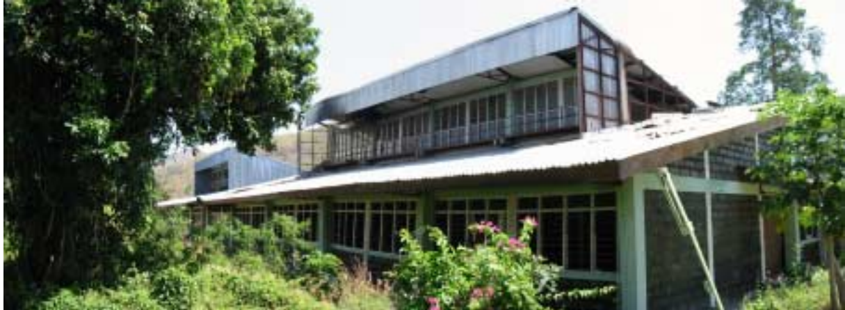
Exterior View: Damaged roof by fire.
