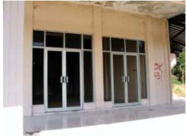
Entrance Aluminum Sash : All glasses are broken.
