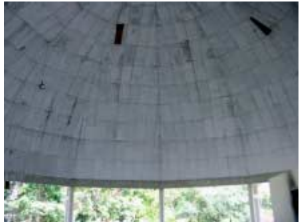
Interior View : Marks of water leakage and fire damage
