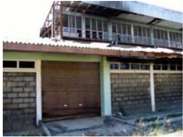
Exterior View : Damaged roof and shutter .
