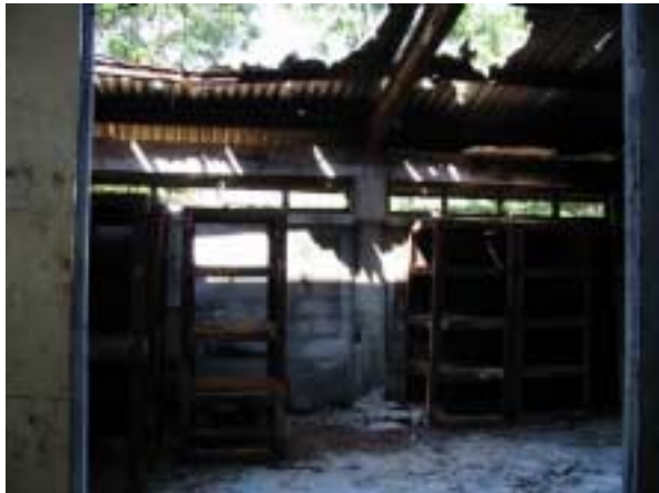
Lower part of Workshop : Roof and ceiling were burnt down.
