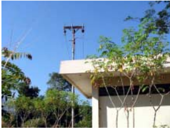
Power intake by aerial electric cable.
