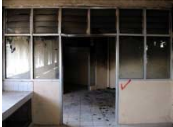
Laboratory : No door panels and aluminum door frame is broken.
