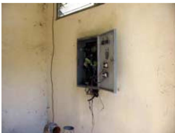
Control board of the lifting pump : broken
