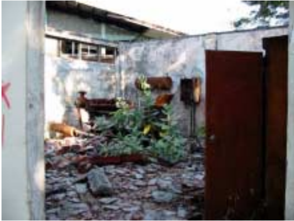
Generator room : destroyed by fire
