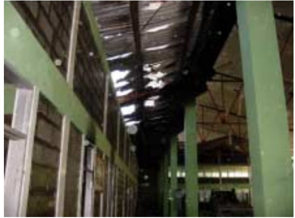
Workshop : Ceiling was burnt down.
