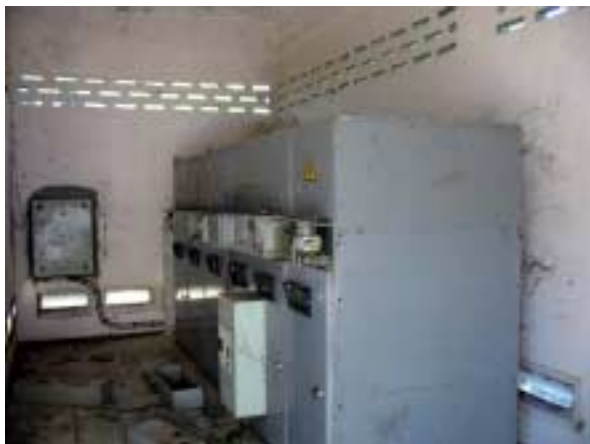
High tension Panel Board was broken intentionally.
