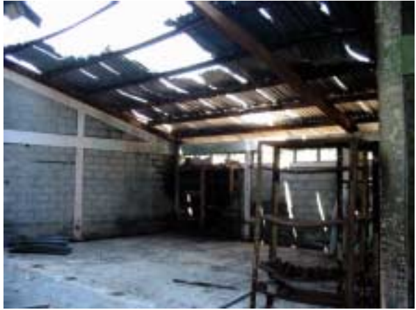
Lower part of Workshop : Fire damage of the roof .
