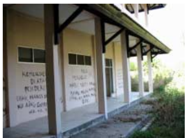
Corridor at the ground floor : Graffiti on the wall.
