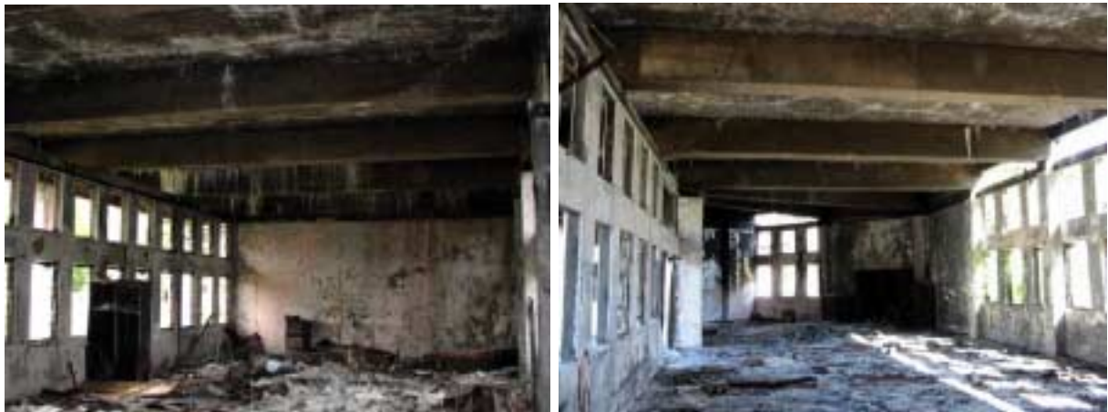
Ground Floor : Fire damage was so severe because there were so many documents to be burnt . Building structure damaged by fire. There were some explosions on the floor slab by fire .
