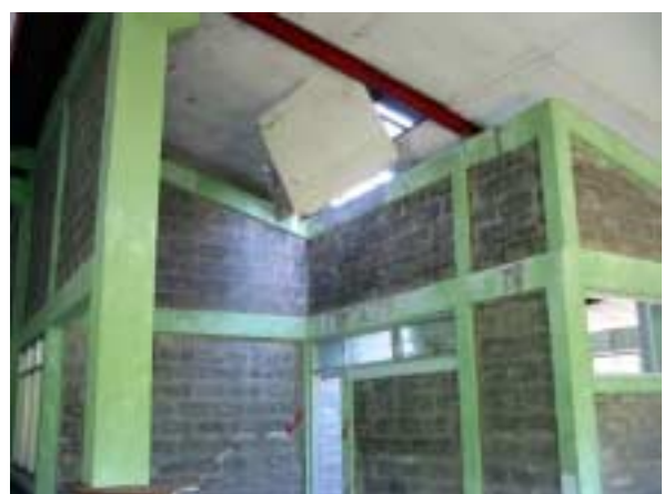
Lower part of Workshop : Broken ceiling and water leakage on the ceiling.
