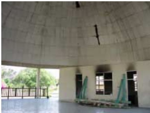
Interior View : Ruins of fire at the kitchen and ceiling
