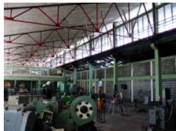
Workshop : Water leakage on the ceiling. Lighting fixtures were removed.
