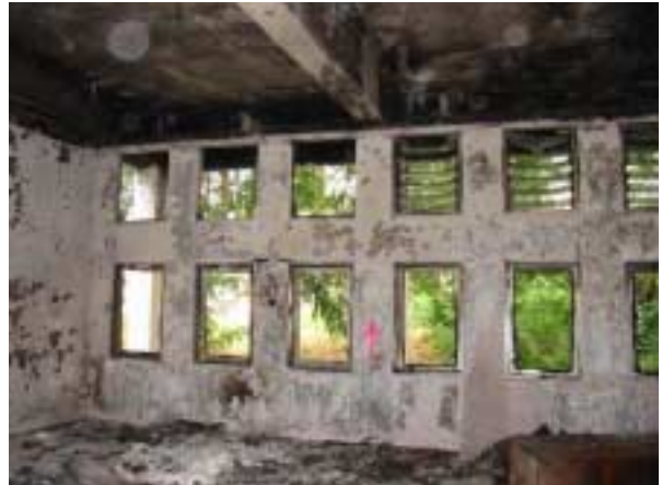
Lecture Room 1-4 : All Finishing coat damaged Sash burnt and bent
