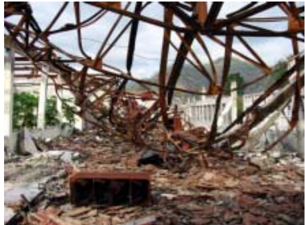
1 st floor classroom : Fallen steel truss
