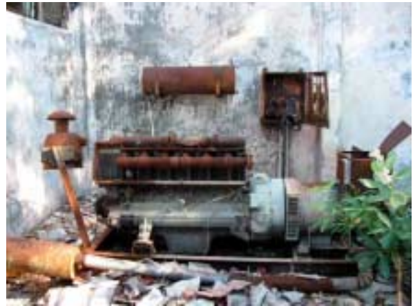
Generator room : burnt switchboard and generator
