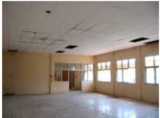
Laboratory : Water leakage on the ceiling.
