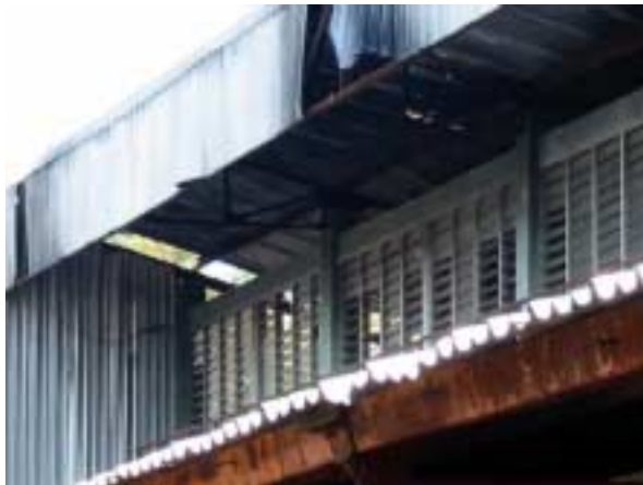
Exterior View : Damaged roof by fire.
