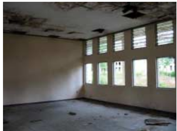
Lecture Room : Water leakage on the ceiling, and wall cracks on the wall.
