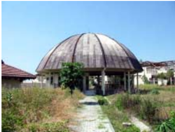
Exterior View : Peeling off the paint
