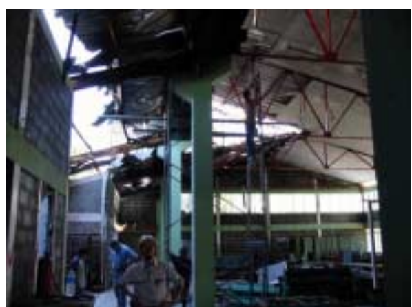
Corridor : Fire damage of the ceiling and roof .
