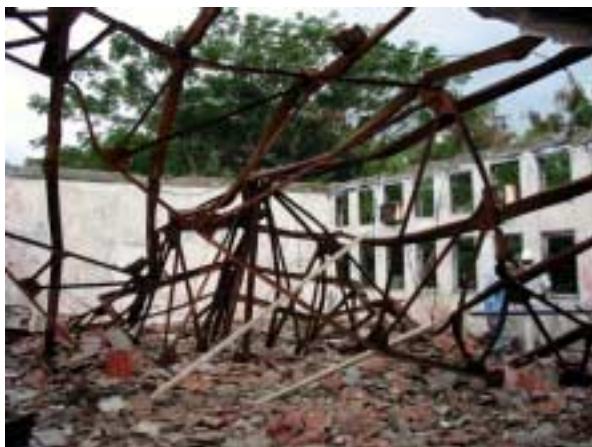
1 st floor classroom : Fallen steel truss
