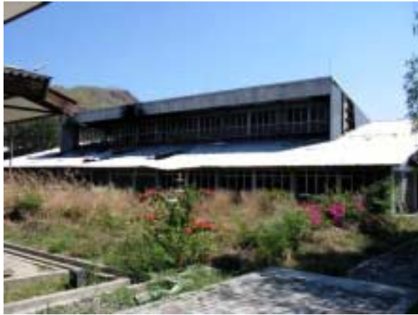
Exterior View : Roof was damaged by fire.
