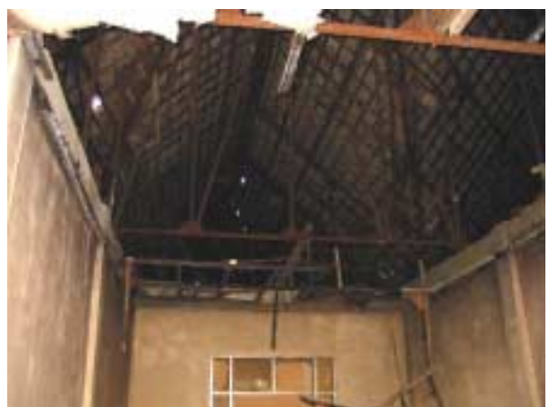
Storage : Ceiling was burnt down. Some roof tiles are removed.
