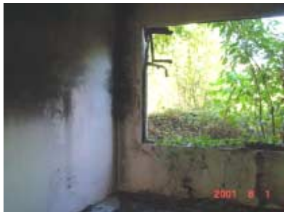
Building C Bed Room :Fire damage Only this room got fire.
