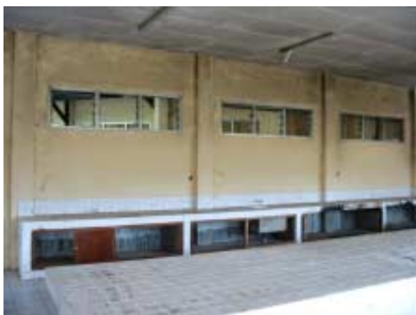
Laboratory : There are fire damage on Floor cabinet.
