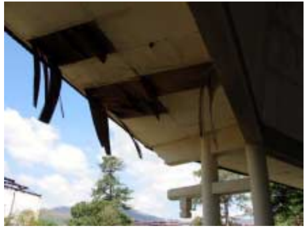
Exterior View : peeled off plywood below eaves.
