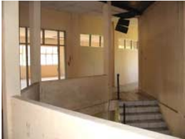
Stair case : Hand rail is missing. Ceiling panel was damaged.
