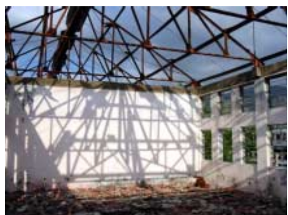
Lecture Room on the 2 nd Floor : Ceiling and roof broken by fire.
