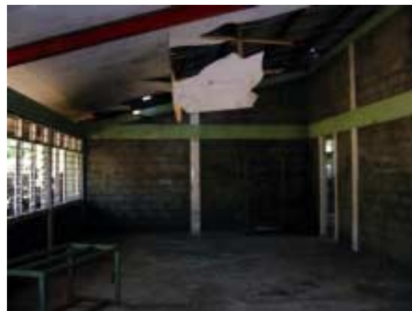
Lower part of Workshop : Fire damaged ceiling.
