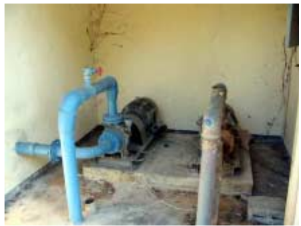
Lifting pump(2,950rpm) : broken
