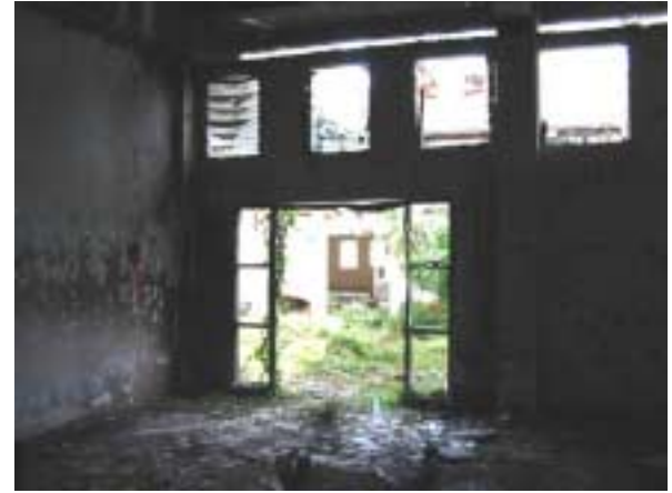
Lecture Room 1-4 : Aluminum sash broken
