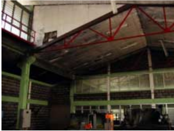
Workshop : Ceiling is damaged.
