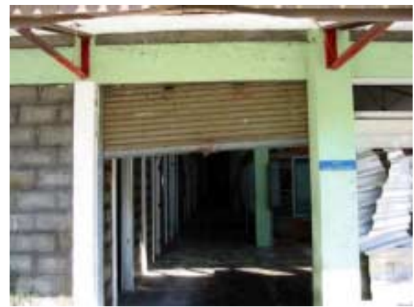
Entrance shutter : It was broken.
