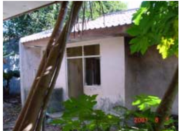
1 story house: It was broken intentionally
