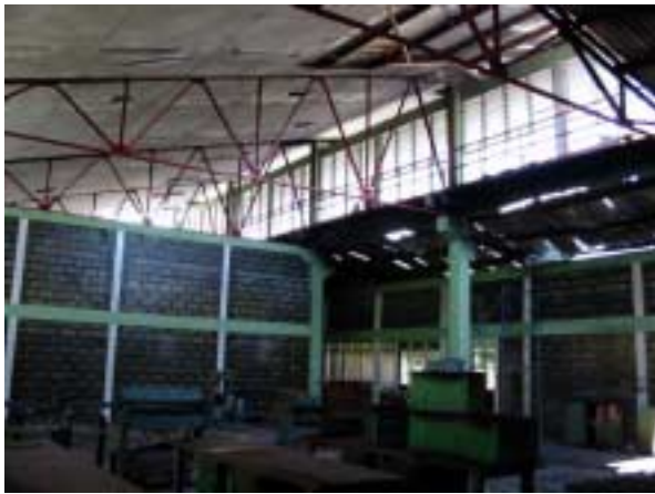
Workshop Interior View : Water leakage on the ceiling.
