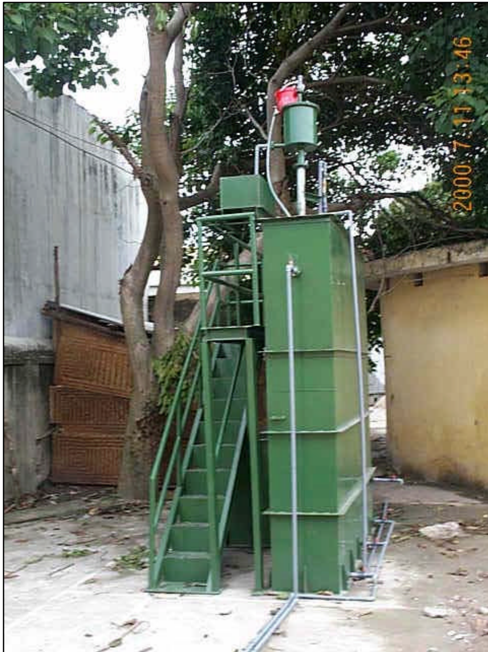
Figure B.5 Picture of the Activated Sludge Plant
