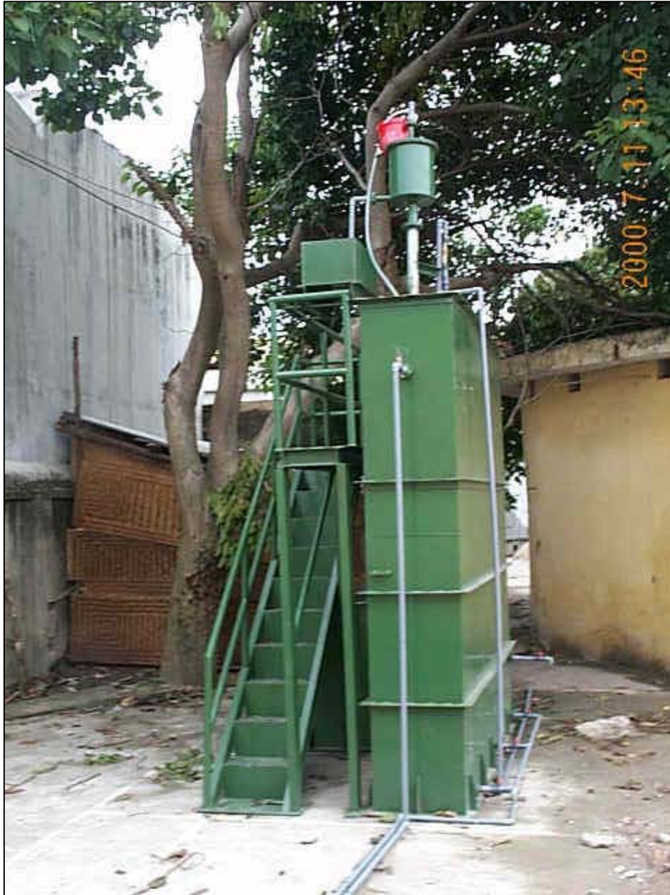
Figure 3.1.5 Picture of Activated Sludge Plant
