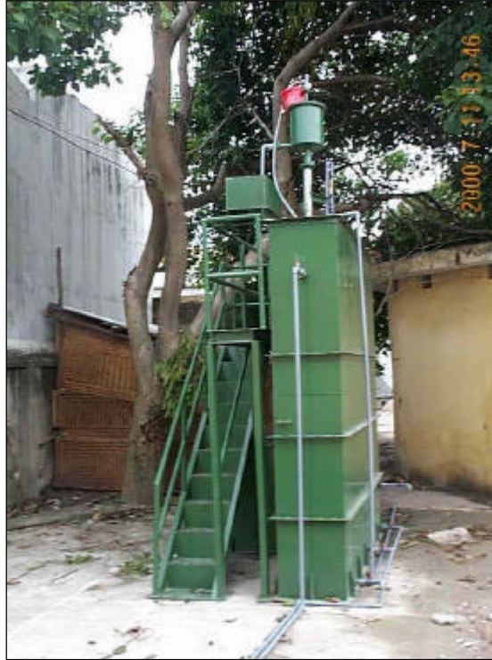
Activated Sludge Process Component
