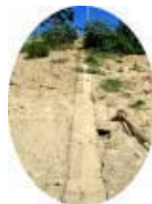
Existing Slope Staff Gauge
