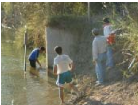
Intake structure of water supply facility
