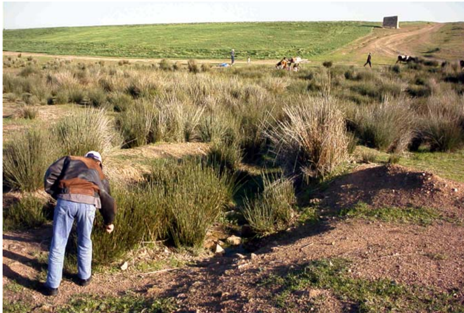
Photo No.12 Damp depression Water level (less than 1m)
