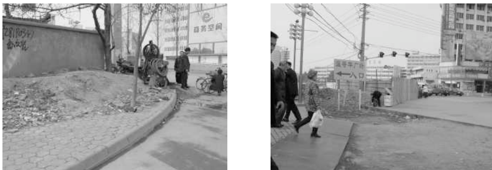
Figure 10.5.9 Waste Soil Piling on Sidewalk and Invasion of Construction Site to Sidewalk
