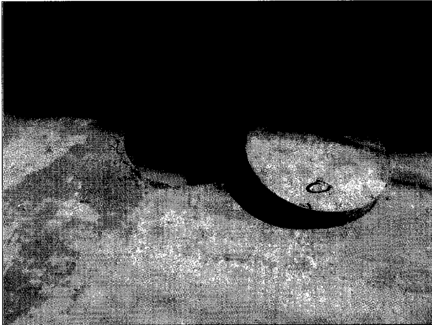
Photo : 7 MODS Zone I Stagnant Sewage at Manhole in Saydabad Area
