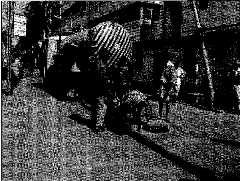
Photo : 11 MODS Zone I Preparation for desludging by Vacuum Truck in Lamin Street
