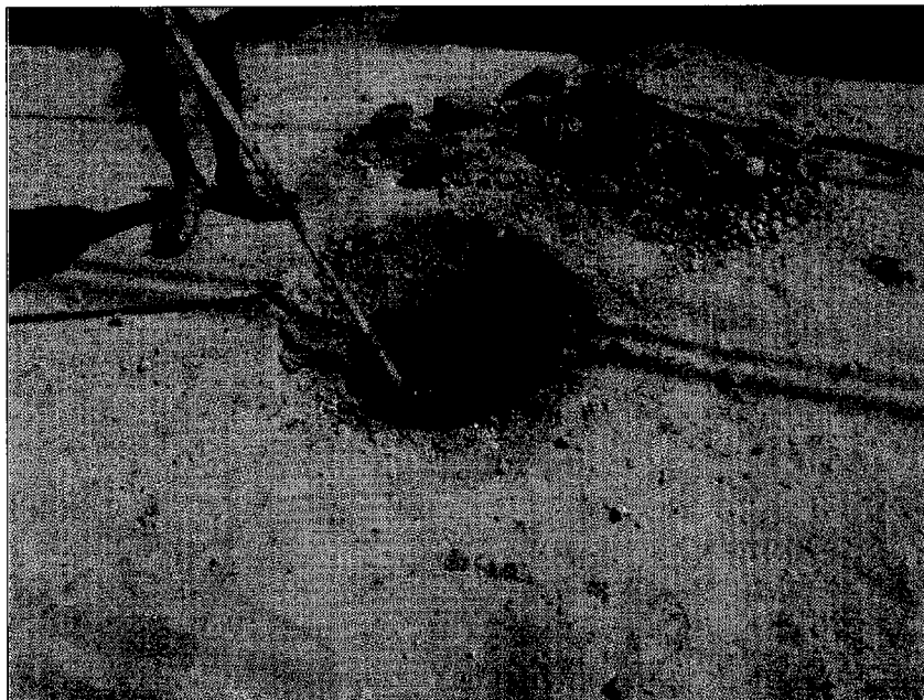
Photo : 6 MODS Zone I Manhole Cover is burried beneath road surface in Saydabad Area.
