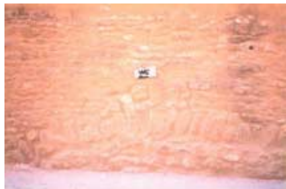
Necessity obliged posting of this crude makeshift sign to complement the one above in a labyrinthine Colosseum. Should be replaced with permanent one.
