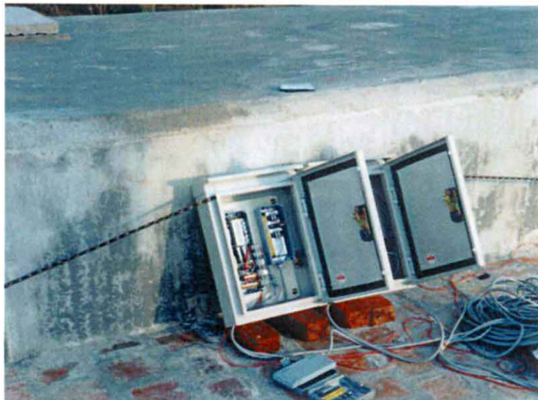
Weather station control unit (data logger)
