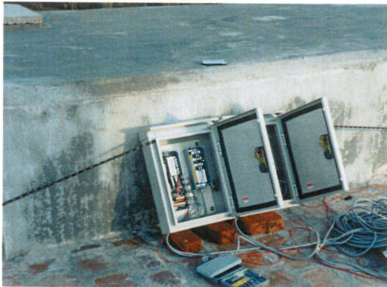
Weather station control unit (data logger)
