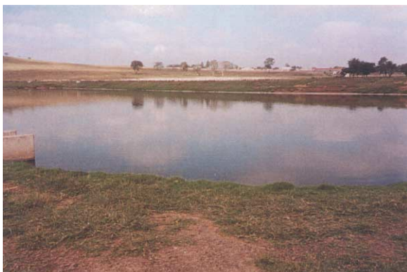
This photo shows a sewerage treatment facility. The construction of this facility was done from the year 1995 to 97 by Japanese donation.
