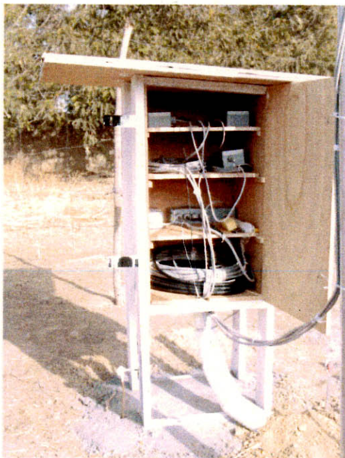
Data logger and battery
