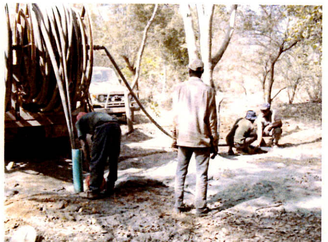
MJMB-E3: Pumping test by air-rift begins. Ground water is coming from the pipe.
