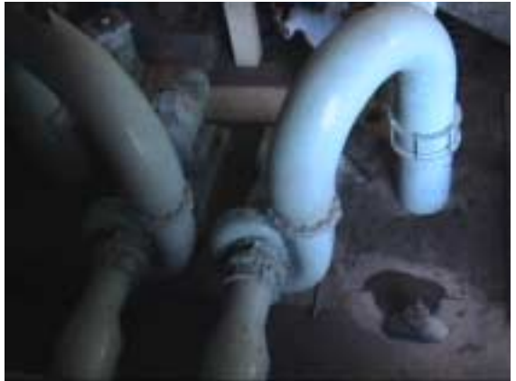
Backwash Pump of Filter and Piping (foot valve is installed on suction pipe)
