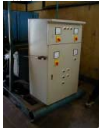
Control Panel for Generator
