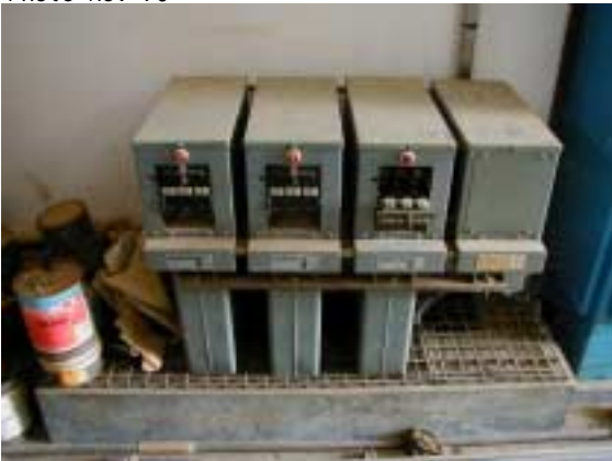
Power Receiving Equipment (condenser)
