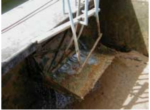
Inlet Gate of Filter (severe stain of gate is observe)
