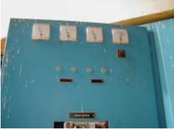
Power Receiving equipment (presently used power receiving panel, front view - 2)
