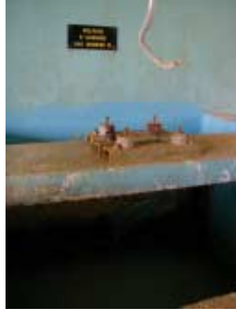
Alum Feeding Equipment (mixer for Alum Solution Tank No2 is removed)
