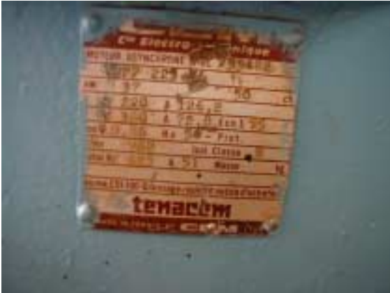
Name Plate of Raw Water Intake Pump
