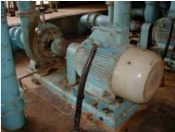
Distribution Pump (reported frequent failure)
