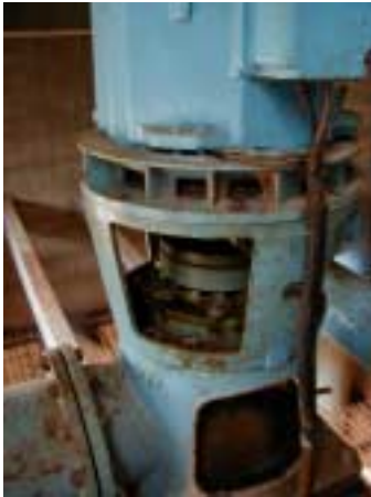
Nake Raw Water Intake Tower, Raw Water Intake Pump and Motor
