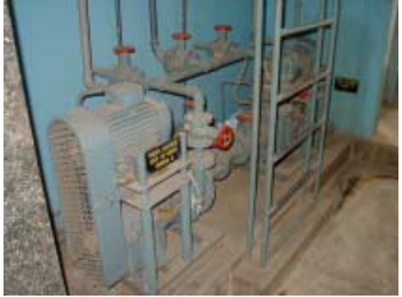
Lime Feeding Equipment (circulation pumps)
