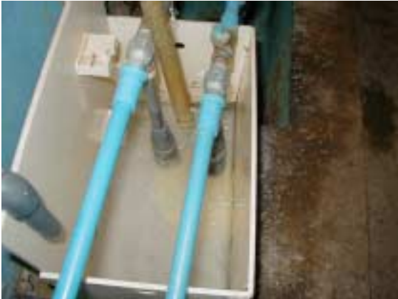
Alum Feeding Equipment (air intrusion into injector is observed due to drop of liquid level)
