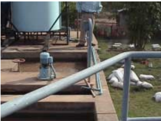
Rapid Mixer on Mixing Well and Piping for Polymer
