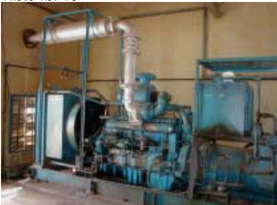
Stand-by Generator (over view)
