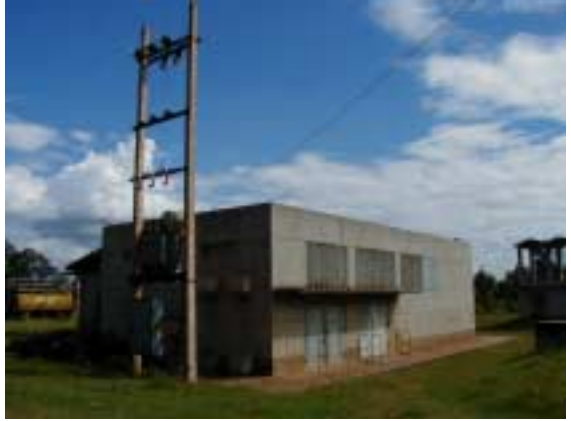
Power Sub-station (over view)
