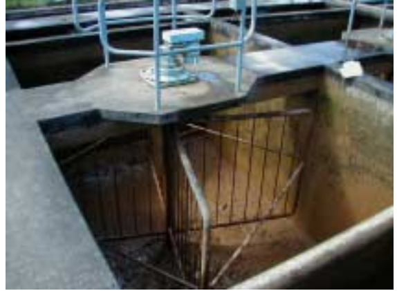
Flocculator (over view)
