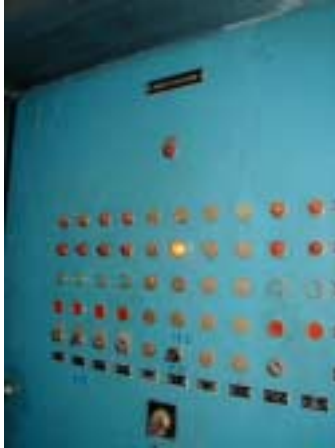
Motor Control Center for Wash Pumps of Sedimentation Basin, Rapid Mixers and Flocculators (front view)
