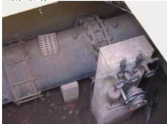
Distribution Header Pipe (Orifice meter is out of order)
