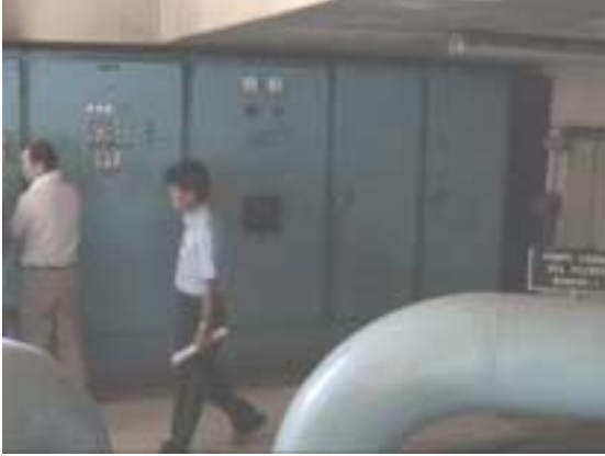
Control Panel of Distribution Pumps (front view - 2)
