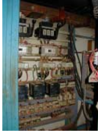
Inside View of Control Panel of Distribution Pumps (deterioration of instrument is observed)
