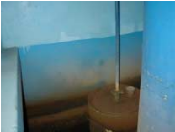
Float for Filter Outlet Control Device (stained)
