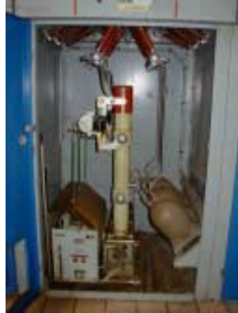
Power Receiving Equipment (power receiving panel, out of order)
