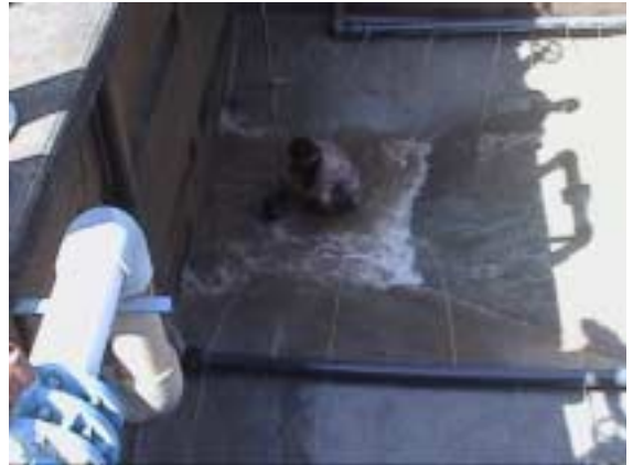
Sludge Valve of Sedimentation Basin (after washing basin operator try to insert valve disk into body)
