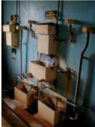
Hypo-chlorite Feeding Equipment (hypo-chlorite feeder)
