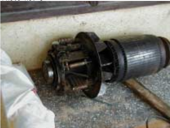
Rotor of Motor for No.3 Raw Water Intake Pump (Rotor has been burnt out)
