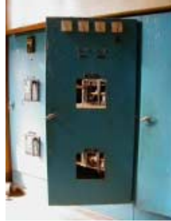
Power Receiving Equipment (presently used power receiving panel, front view - 3)
