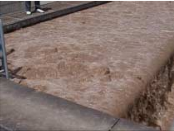
Be in Filter Washing (damage of filter under drain is suspected from air blowing at the inlet of filter)
