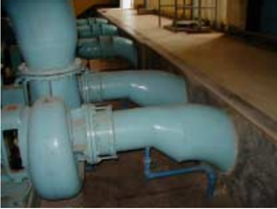
Backwash Pump of Filter (priming pipe for suction pipe is connected with delivery header main)
