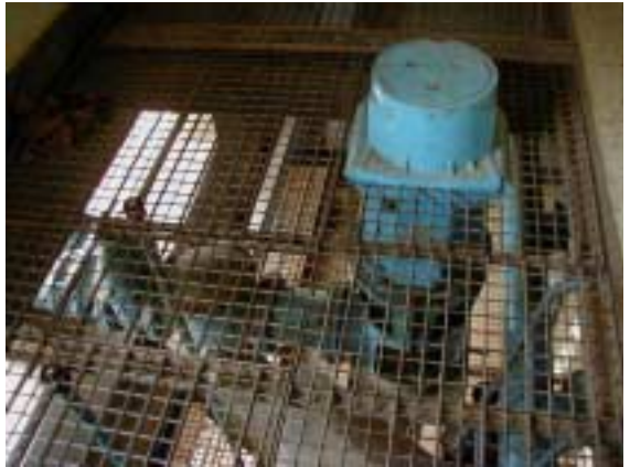
Nake Raw Water Intake Tower, Raw Water Intake Pumps and Floor with Grating
