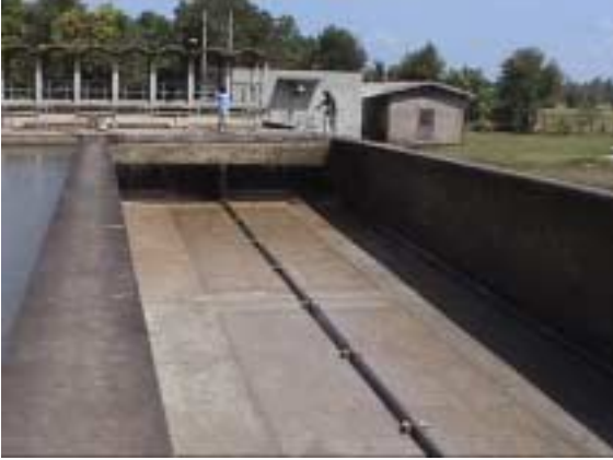
Wash Pipe of Sedimentation Basin
