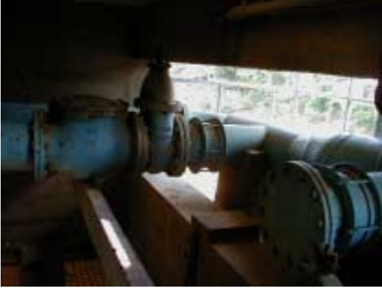
Nake Raw Water Intake Tower, Raw Water Intake Pump and Piping -1
