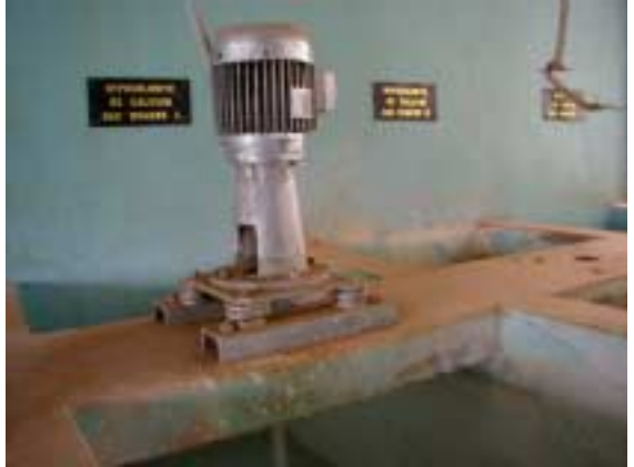
Hypo-chlorite Feeding Equipment (only one solution tank is used)
