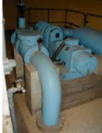
Air Blower of Filter
