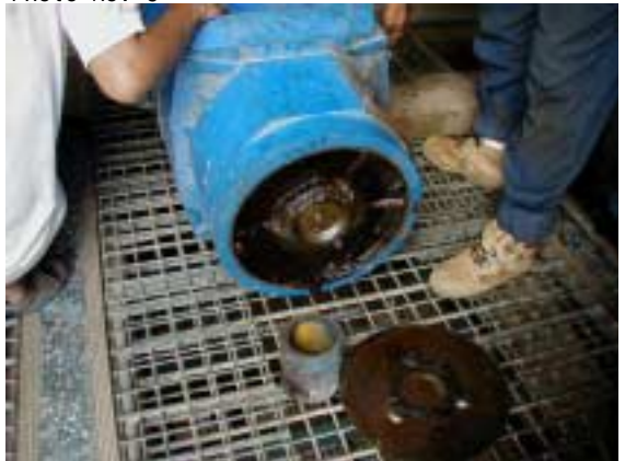
Motor Failure for No.3 Raw Water Intake Pump due to over lard (on 24 Oct'2000)
