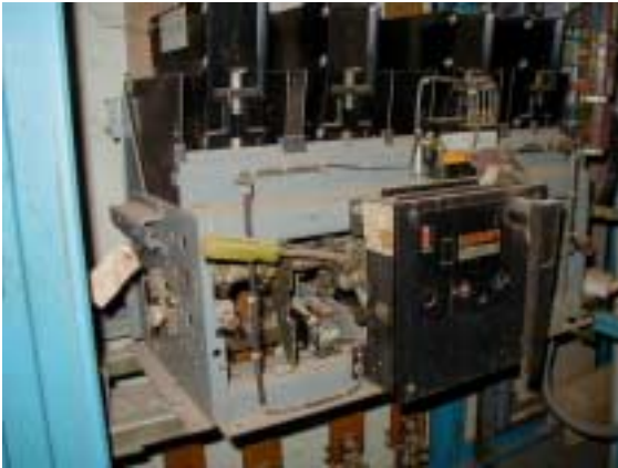
Inside View of Control Panel of Distribution Pumps (screwdriver is used for switch gear lever)
