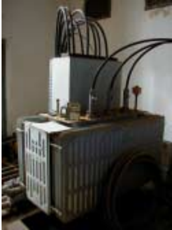
Power Receiving Equipment (transformer, out of order)
