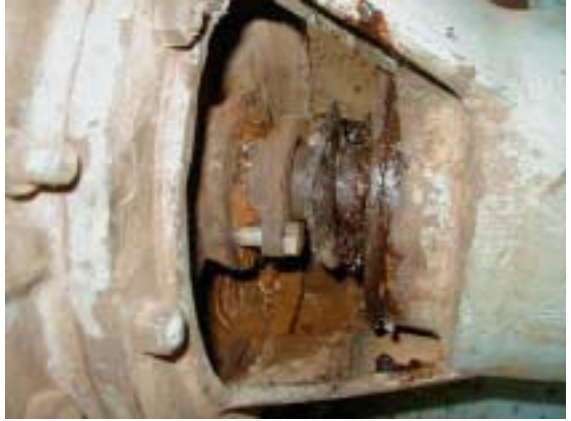
Distribution Pump (severe stain is observed on gland)
