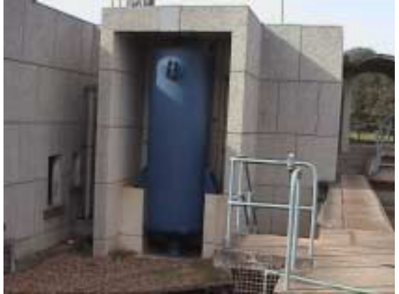
Air Chamber for Surge Control
