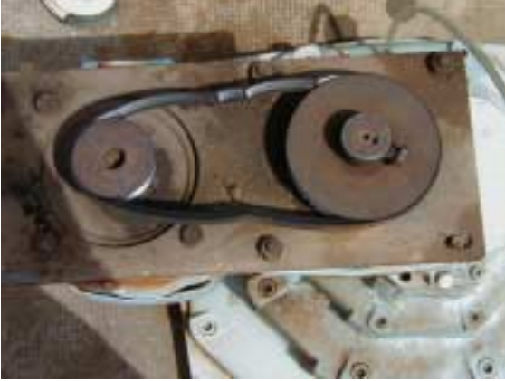
V-Belt of Flocculator (belt is being cut)
