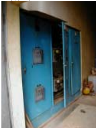
Power Receiving equipment (presently used power receiving panel, front view - 1)
