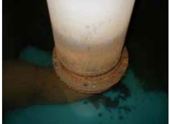
Filter Outlet Control Device (controller under water is stained)
