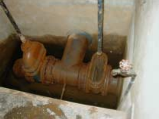
Outlet and Backwash Valve (stained)
