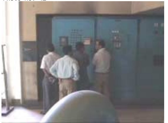
Control Panel of Distribution Pumps (front view - 1)
