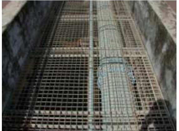
Raw Water Transmission Main on Operation Bridge (spiral SP with dresser joint)
