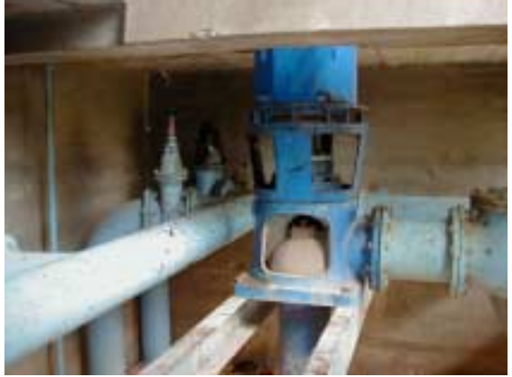
Nake Raw Water Intake Tower, Raw Water Intake Pump and Piping -2
