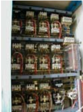
Control Panel for Chemical Feeding Equipment (inside view of panel)
