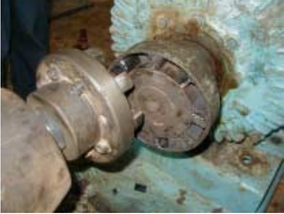
Distribution Pump (rubber pad for shaft coupling is Damaged frequently)
