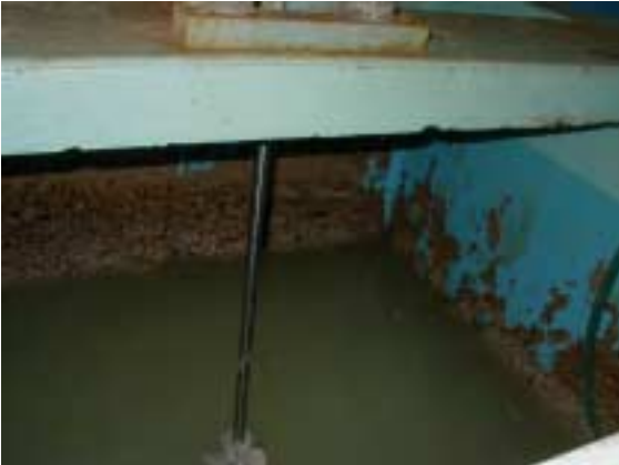
Hypo-chlorite Feeding Equipment (severe deterioration is observed on interior surfaces)
