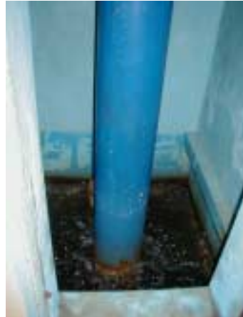
Filter Outlet Control Device (over view)
