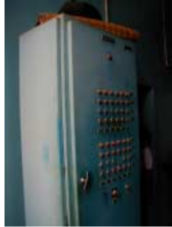
Control Panel for Chemical Feeding Equipment (front view, out of order)
