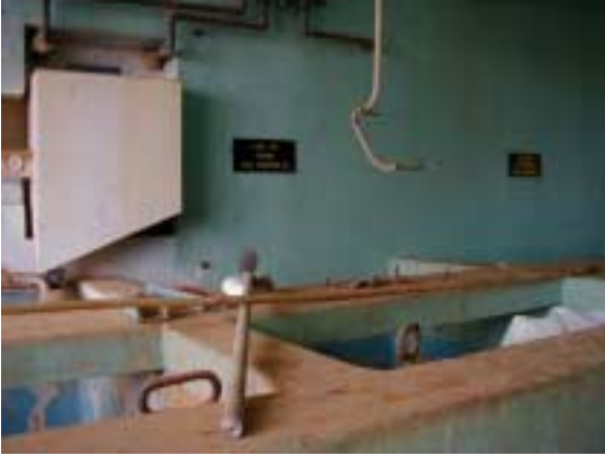
Lime Feeding Equipment (mixers on solution tanks are removed)
