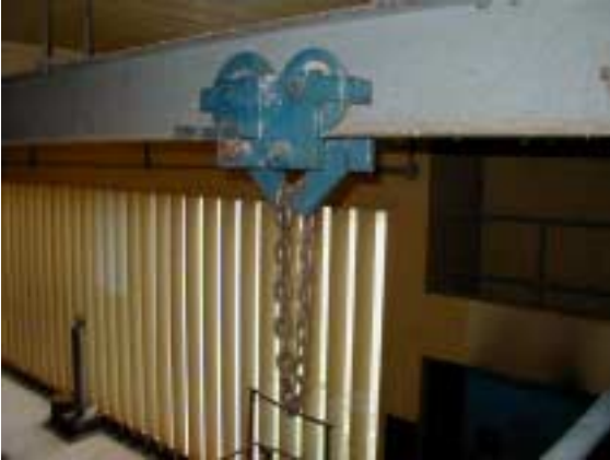
Monorail Hoist in Distribution Pump Room (hoist crane is out of order)
