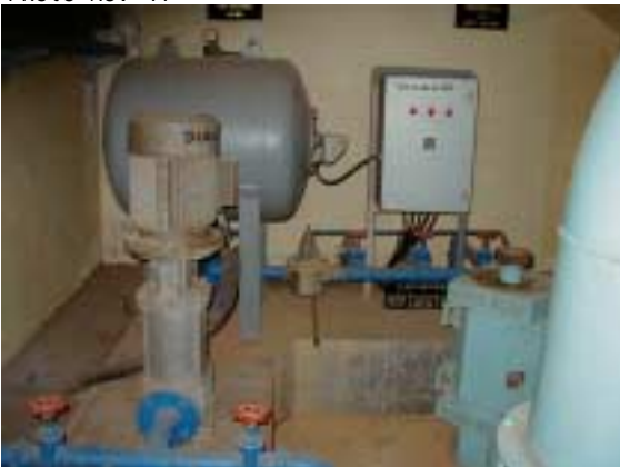
Air Compressor for Air Chamber (out of order)
