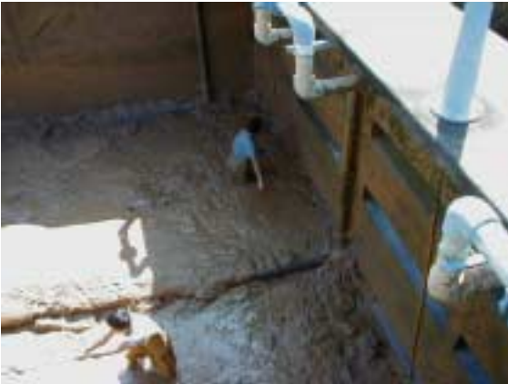
Sludge Valve of Sedimentation Basin (bent valve shaft with stain)
