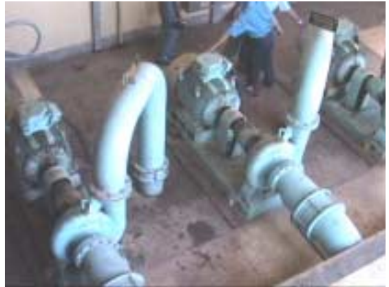
Distribution Pumps and Piping (vibration of discharge pipe is observed due to no support)
