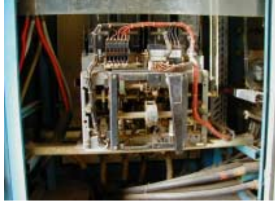
Power Receiving Equipment (inside view)
