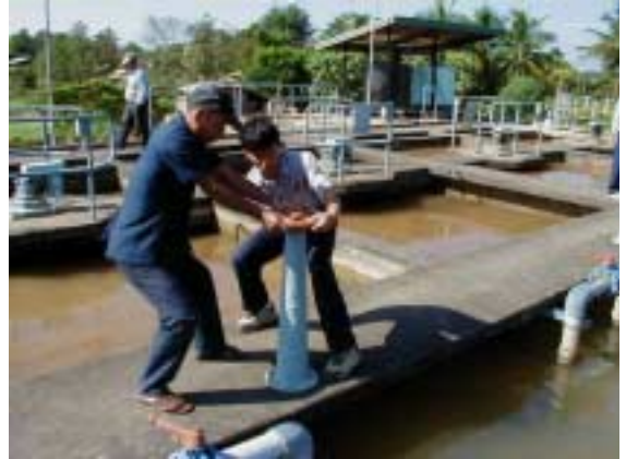
Operating Floor Stand for Sludge Valve of Sedimentation Basin (two operators try to open the valve)
