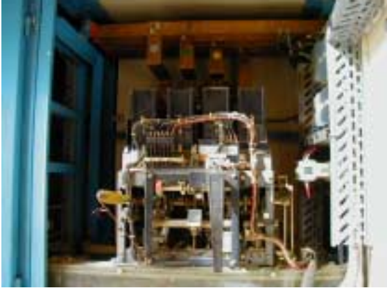
Power Receiving Equipment (inside view, screwdriver is used for switch gear lever)
