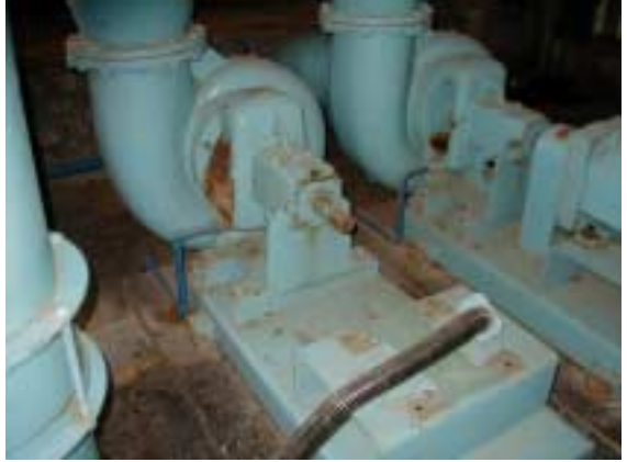
Backwash Pump of Filter (Motor is out of order)
