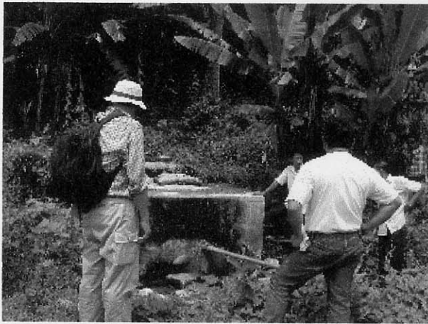
Intake Box of Existing Level-2 System
