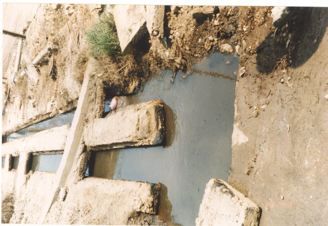
Photo. MRC-2 Wastewater Sewer
