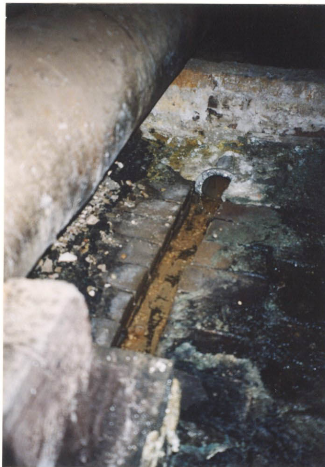
Photo. EIS-4 Leakage (Acid) Water Sewer
