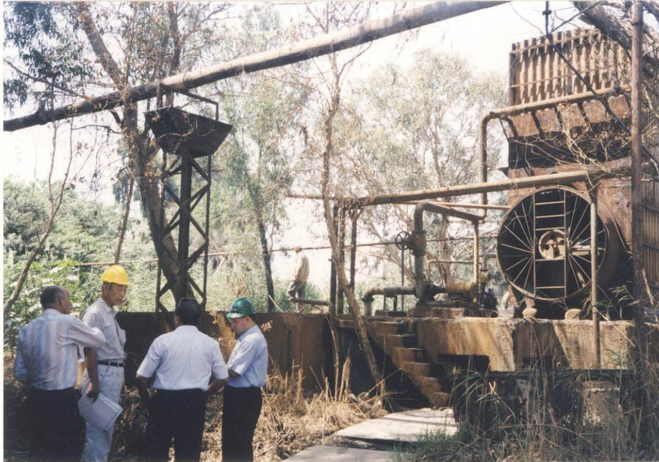
Photo. MRC-3 Old Type Cooling Tower
