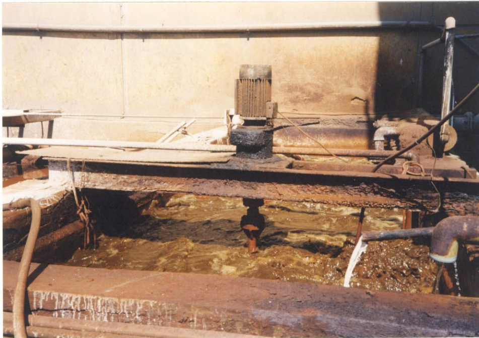
Photo, NSP-3 Neutralization Plant for Pickling Wastewater
