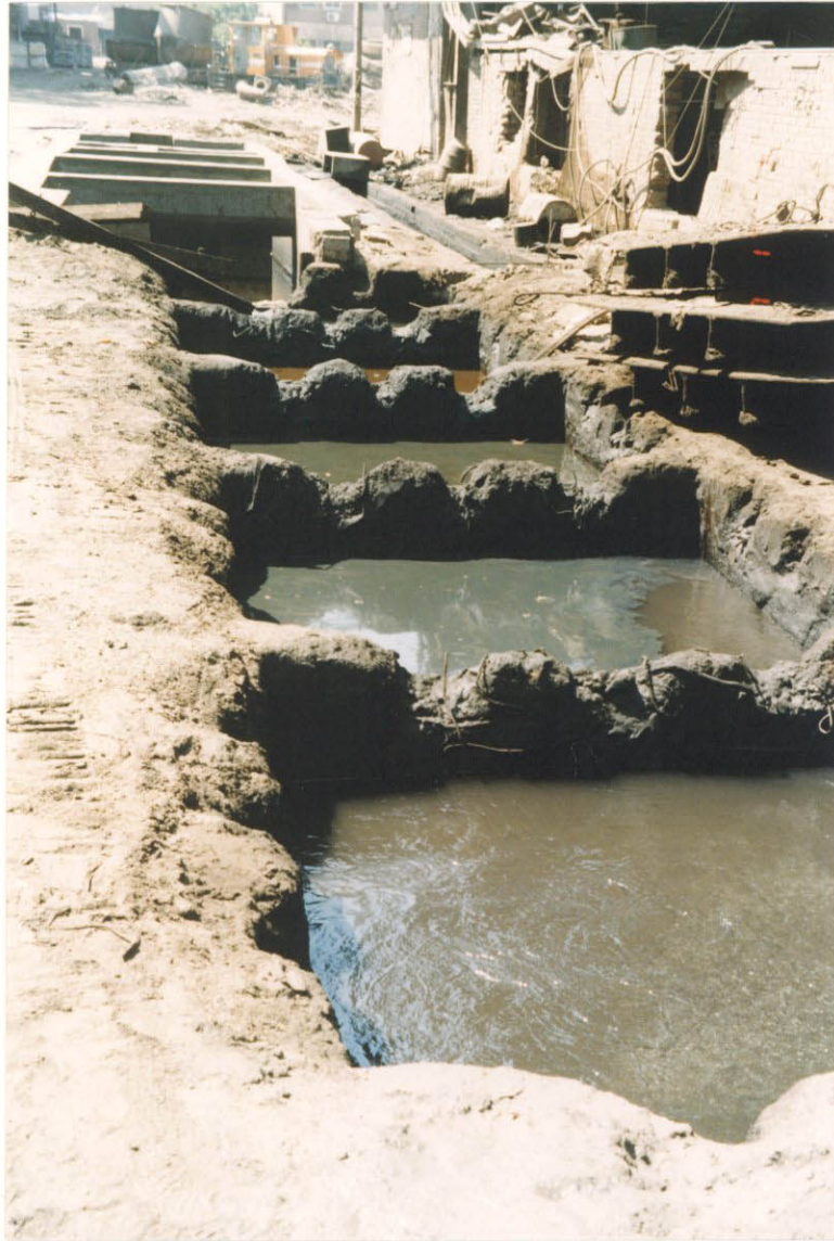
Photo. DSM-1 Oil Trap of Wastewater Sewer
