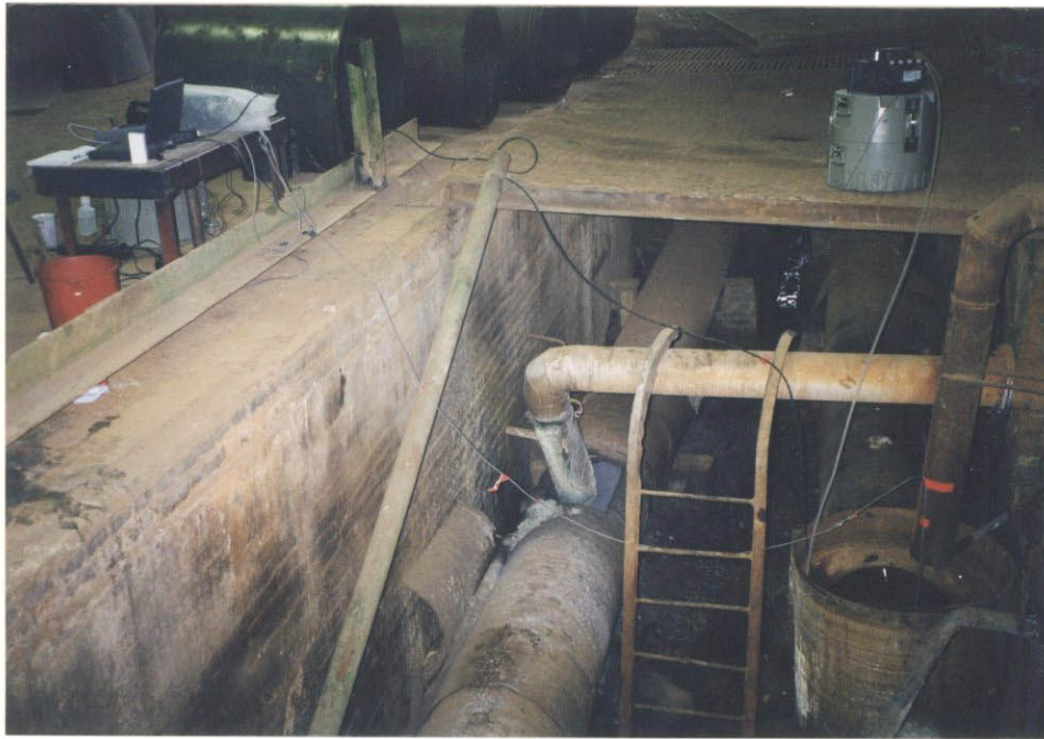
Photo. EIS-3 Sampling Points Left: Spent Sulfuric Acid Pipe Right: Rinsing Water
