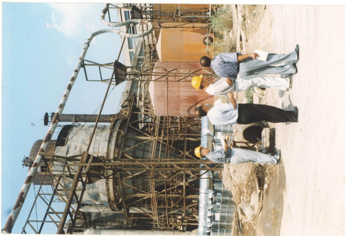
Photo. MRC-1 Resin Plant Constructed by SUMITOMO Japan.
