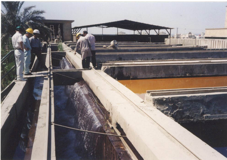
Photo. NSP-4 Oil Separator Basin for Cooling Water
