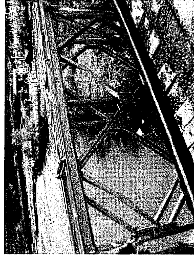
Members were bent at several places.
