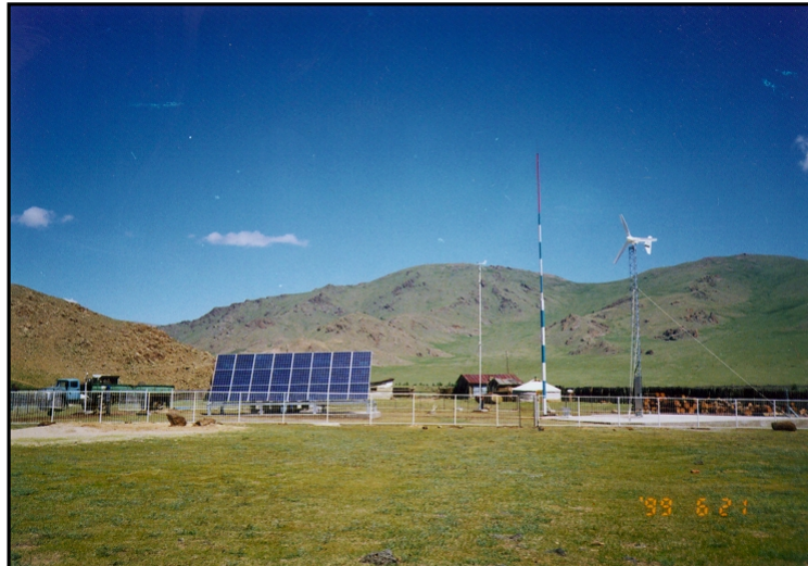
Photo II.2.1-1 Pilot Plant in Tariat Sum
