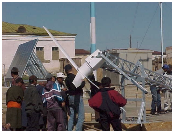
Photo II.1-8 Completing the Assembly of Wind Turbine and PV Array
