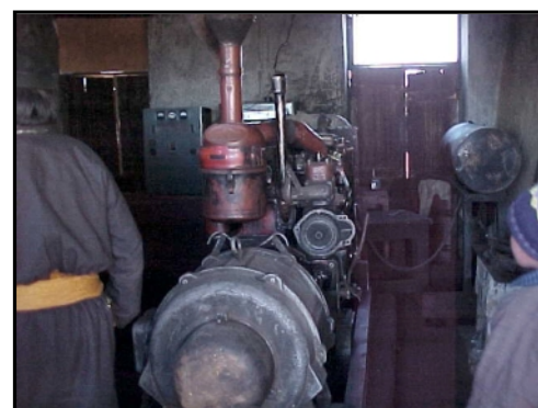
Photo I. 7. 4-2 Russian Diesel Generator in Uulbayan Sum Center
