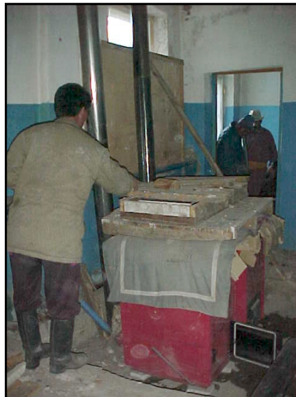
Photo I.7.9-3 Boiler for Individual Central Heating System (Natural Circulation)
