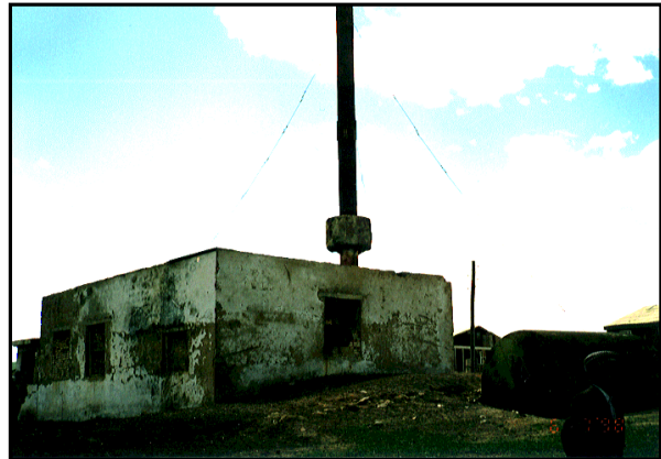
Photo I.7.9-1 Boiler House of Central Heating System (Naran Sum Center of Sukhbaatar Aimag)
