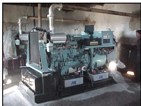
Photo I. 7. 4-3 Japanese Diesel Generator in Sevrei Sum Center
