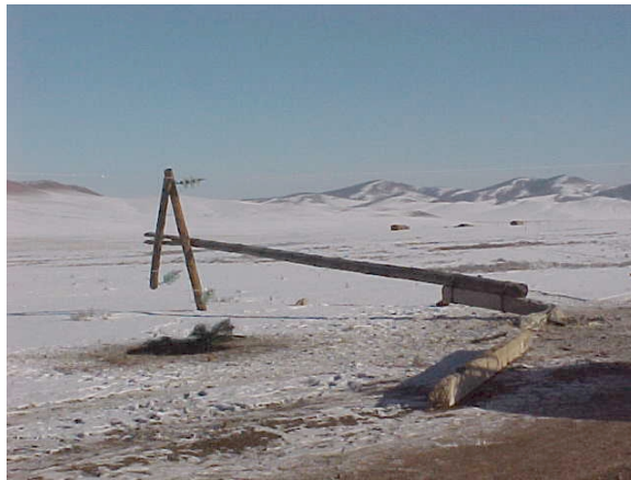
Photo I.5.3-1 35 kV Transmission Line Pole fallen down by Traffic Accident
