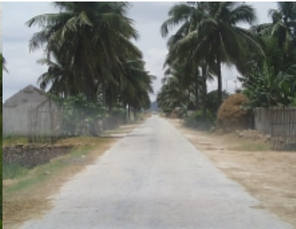
National Highway 91, Can Tho Province in Suburban Area of Can Tho City
