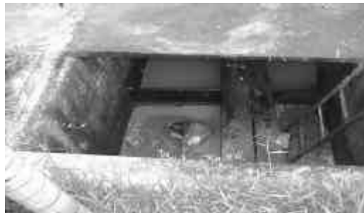
Figure 4 Oil Separator at the final discharge point for wastewater
