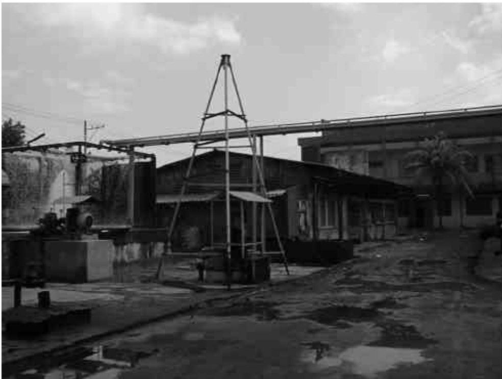
Food Factory / Cooling Process for Recovered Cooling Water
