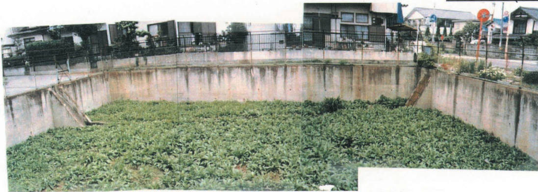
Hutatuya Detention Pond, Kitamoto city, Saitama (Built in 1981)
