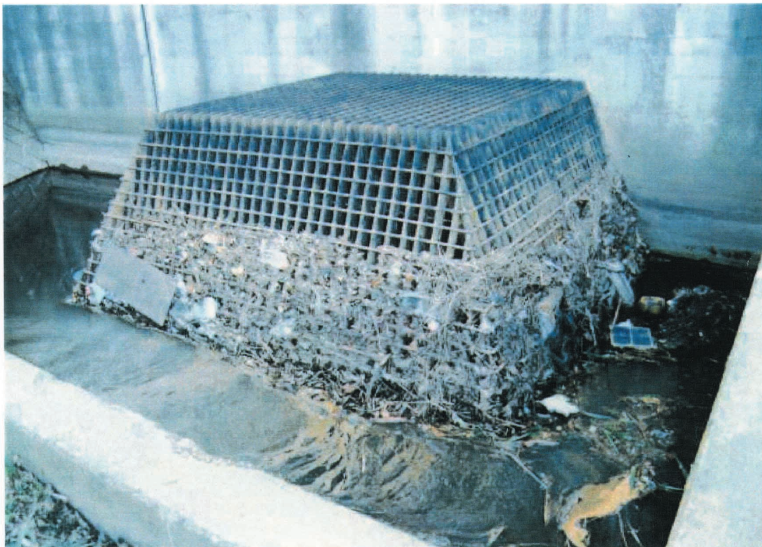
Outlet Screen of Hinatayama Detention Pond
