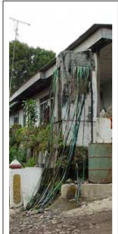
Photo Distribution box
