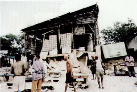
Photo 3: Old Ice Plant The foundation was scoured by waves.
