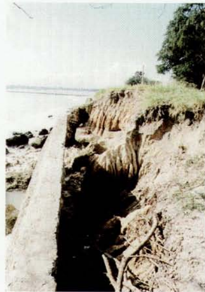
Photo 2: Revetment near Point-A Sand inside was scoured.
