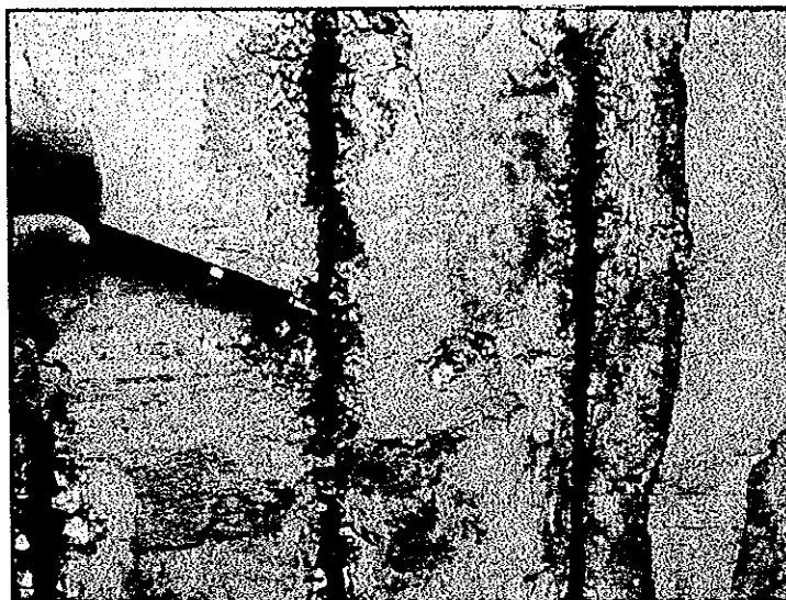
Inadequate cover and corrosion of reinforcement
