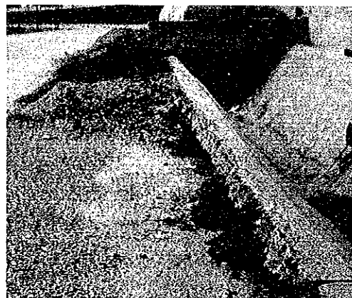
Subsidence of Shoulder at Embankment
