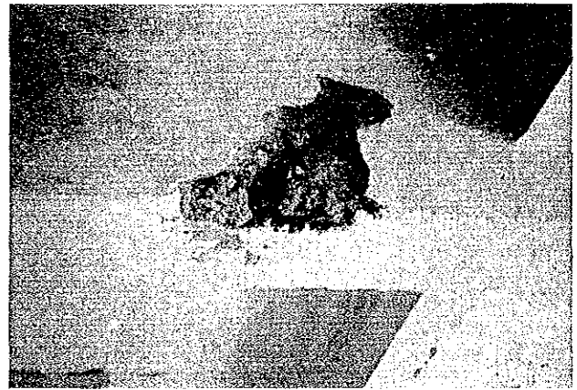
Photo 3.11.31 Concrete cover spalled and main re-bars exposed in beam (the splice of main bar is exposed and cover concrete around the hook dropped off.)
