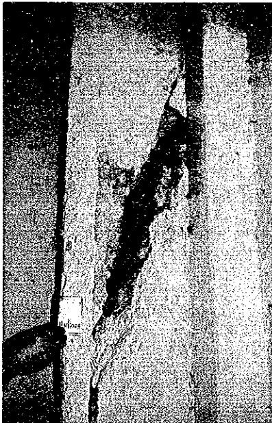
Photo 3.11.36 Shear failure occurred in column of the above building
