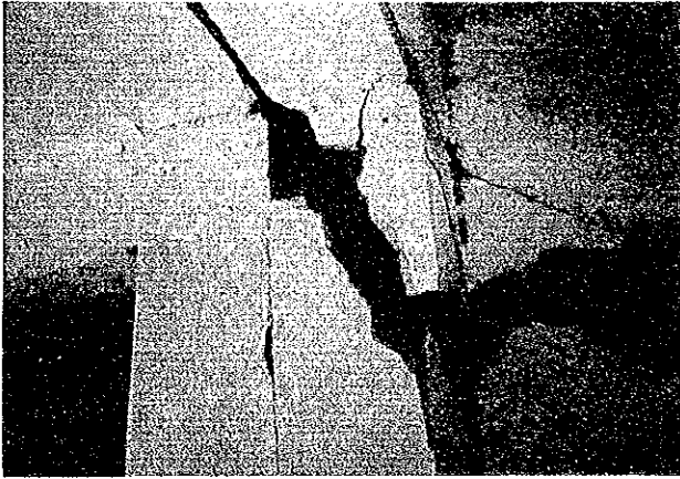
Photo 3.11.34 Shear failure of column facing expansion joint (lateral re-bars cannot be seen)
