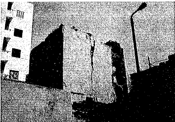
Photo 3.11.5 Non-reinforced masonry building (walls fell off out-of-plane)
