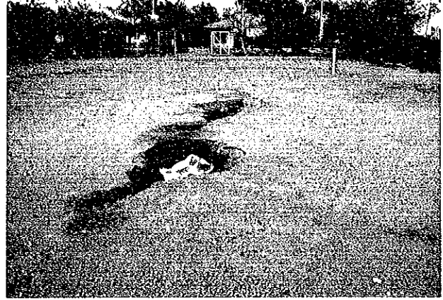
Photo 6.8 Soil Liquefaction Maumere Port Port facility. Paved area was damaged. In this case, sand boils came out from cracks by soil liquefaction.
