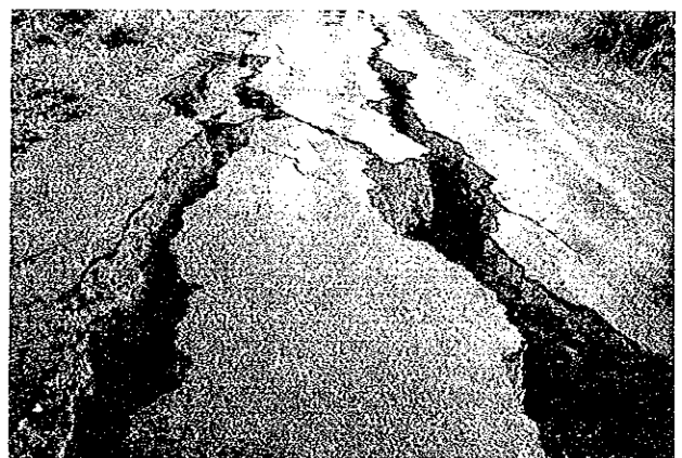
Photo 5.18 Cracks on Pavement
