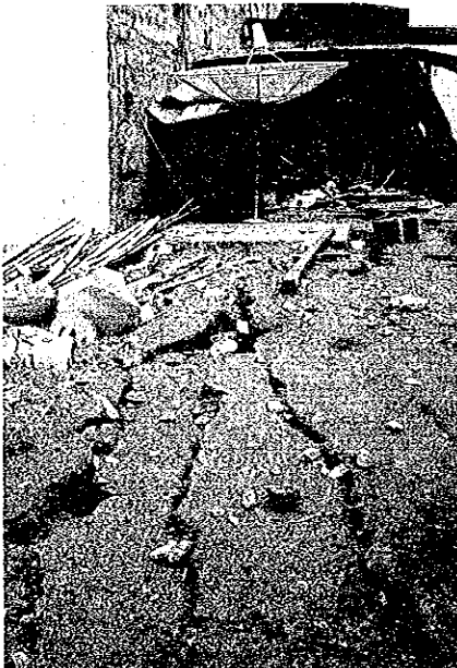
Photo 5.46 Cracks along the Coast (Maumere City)
