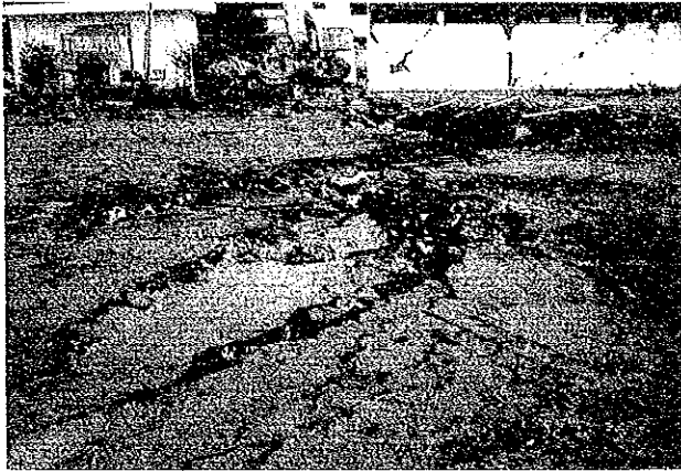
Photo 5.30 Settlement of Pavement due to Soil Liquefaction
