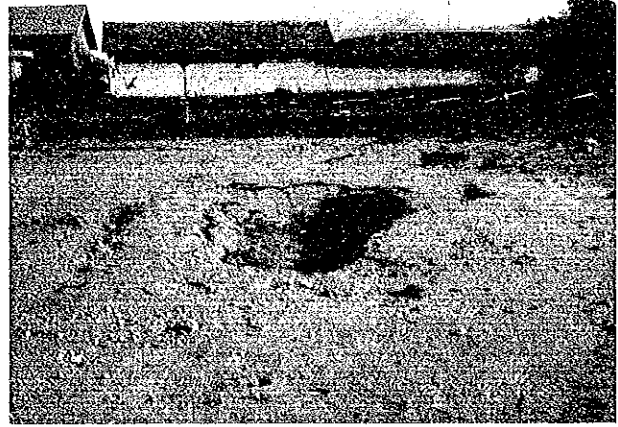
Photo 5.31 Cracks and Settlement of Pavement due to Soil Liquefaction
