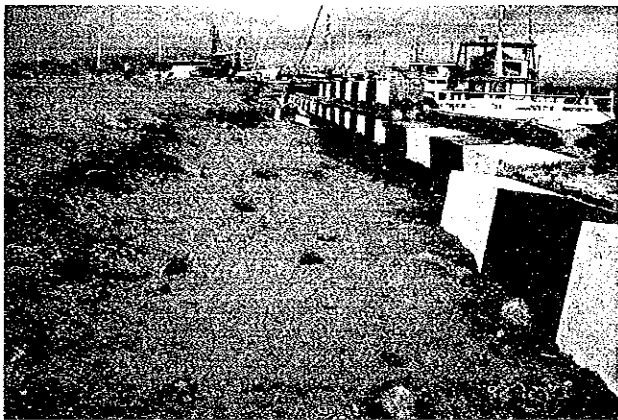
Photo 5.27 Tilting of Retaining Wall and Settlement of Back-Fill
