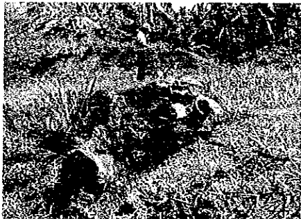
15. Culvert Damage (CLV - D) Spot L - 81 (Leyte)
