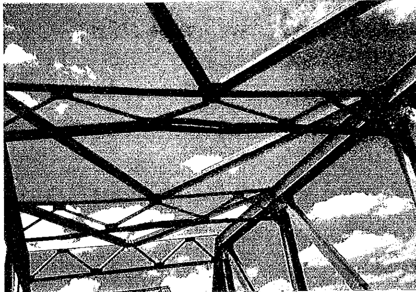
Photo. 5-4. Severely Bent Bracings
