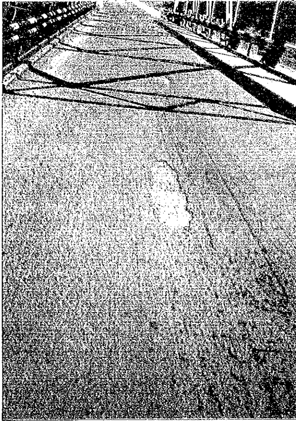
Photo 5-5. Pot Holes on Carriageway
