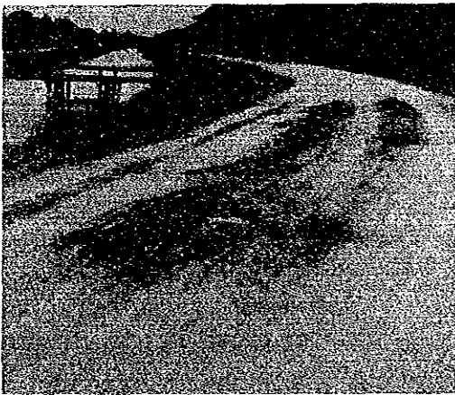
IM-11 Typical View
