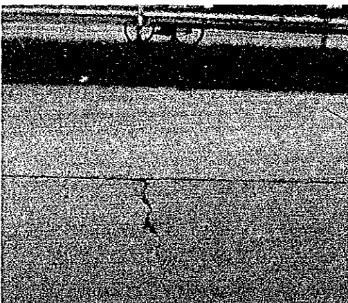
Transverse Cracks on Concrete Pavement (Rt. 34)
