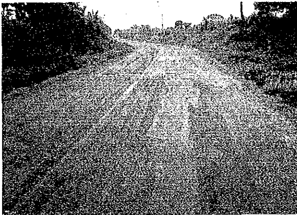
DBST pavement in "fair" condition P19-2: Gen. Trias-Amadeo
