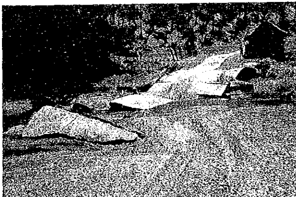
Collapsed spillway B0-1: Malinta-Lagta, Barangay road, Masbate
