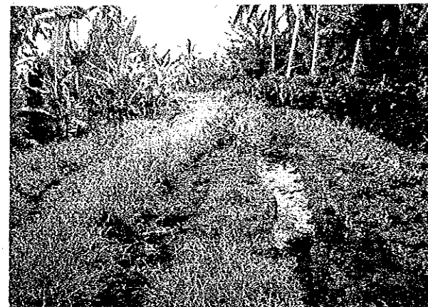
Earth road in "impassable" condition B9-4: Panukan Gubat Road
