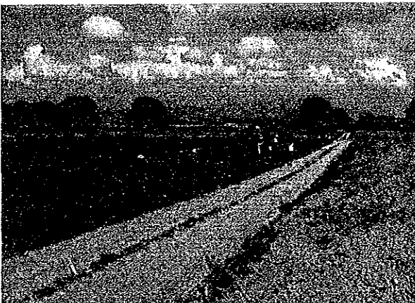
Earth road in "bad" condition B9-3: Palindong Road
