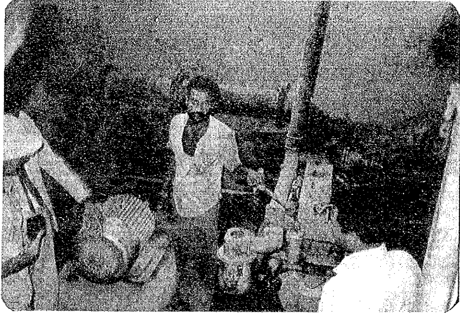
Photo 2.9 Existing Pumping Station (Bilbeis)
