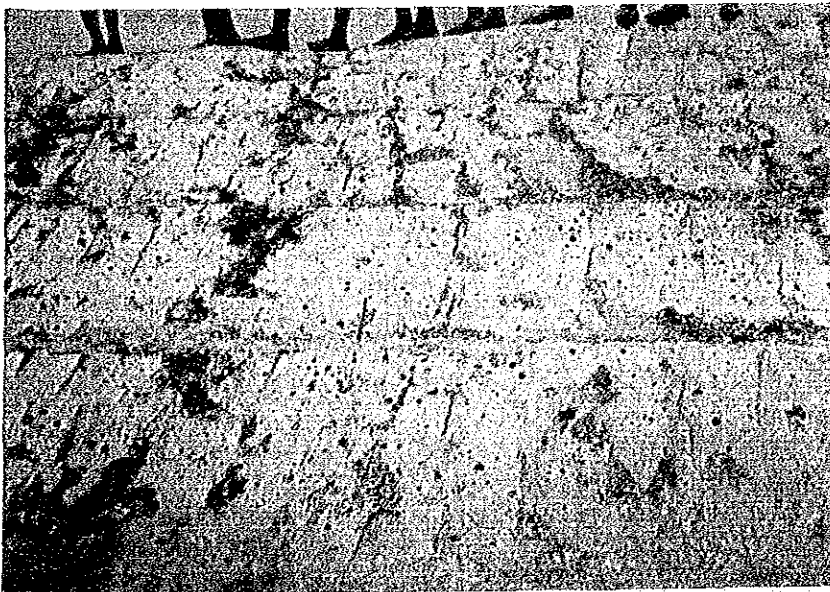
Many holes found in the existing embankment body during the emergency work (made by some kind of insect)
