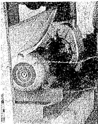
Irrigation Pump for the Project
