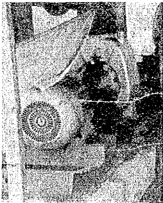
Irrigation Pump for the Project
