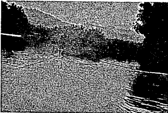
Poigar River, Bridge was washed away. 74.5km from Kotamo-Bagu.
