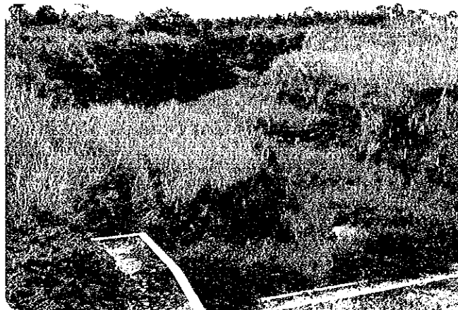
Photo-15 Lower reach of K.Besuk Sat No.1 Sabo Dam before the disaster on May 14th. This dam is situated quite important point from where Besuk Sat Lama is diverted. And this dam showed its big effects this time stopping the Lavar to Lumajang.
